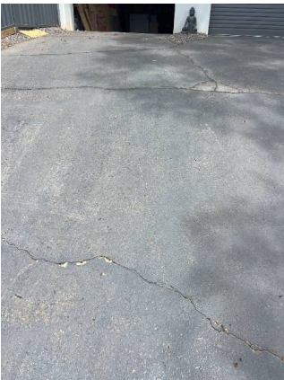
Cracks in driveway.
