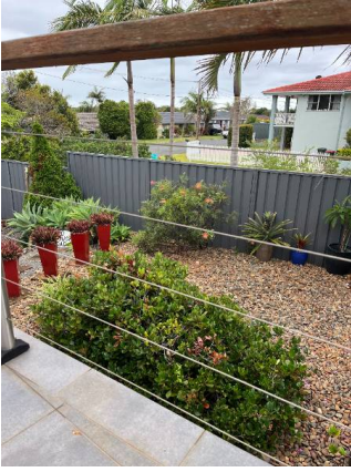
Wire balustrade is loose.
