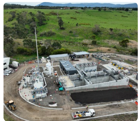
Gisborne Recycled Water Plant
