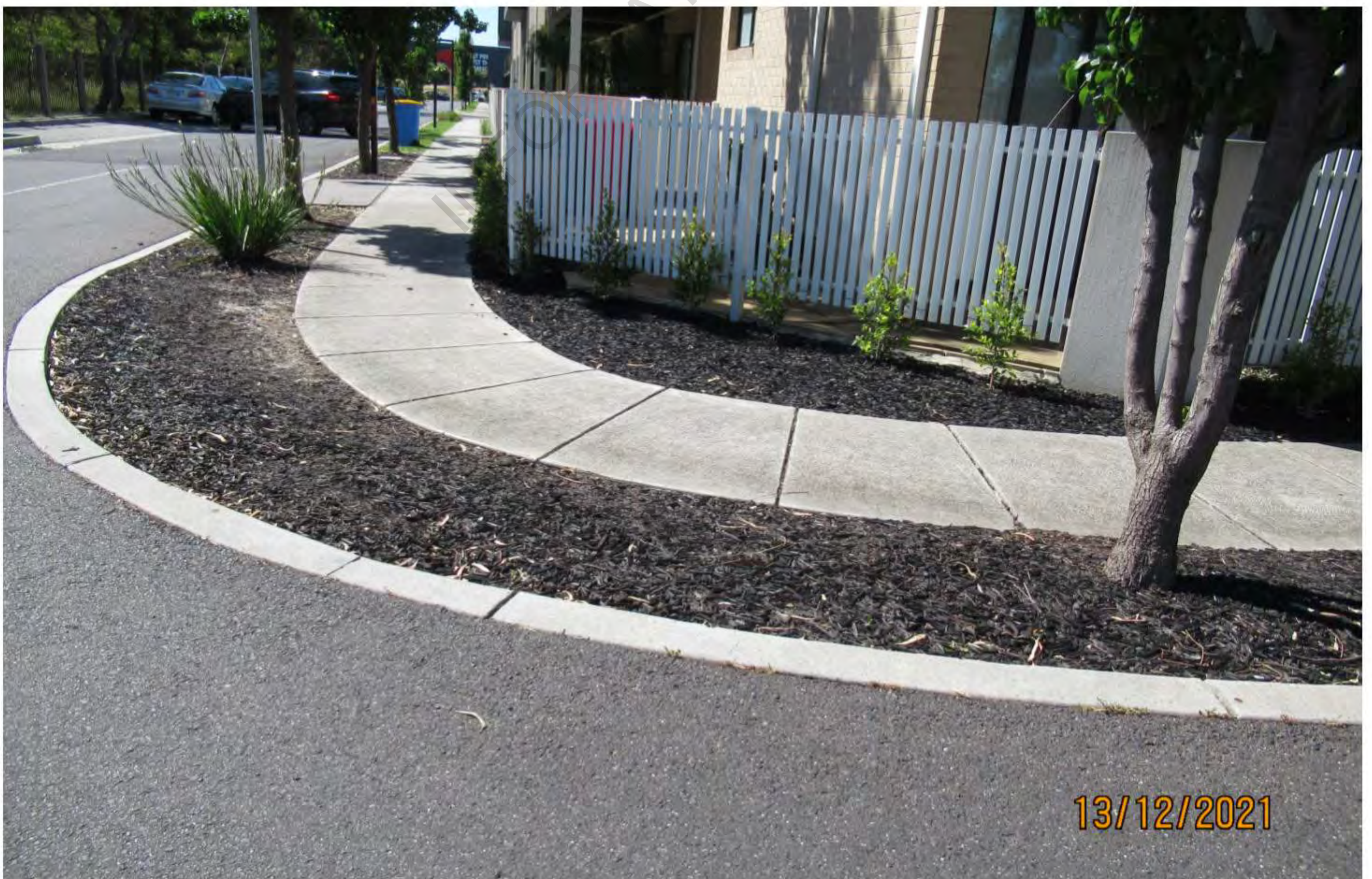
Photo 1.20: Concrete footpath has subsided in various areas
