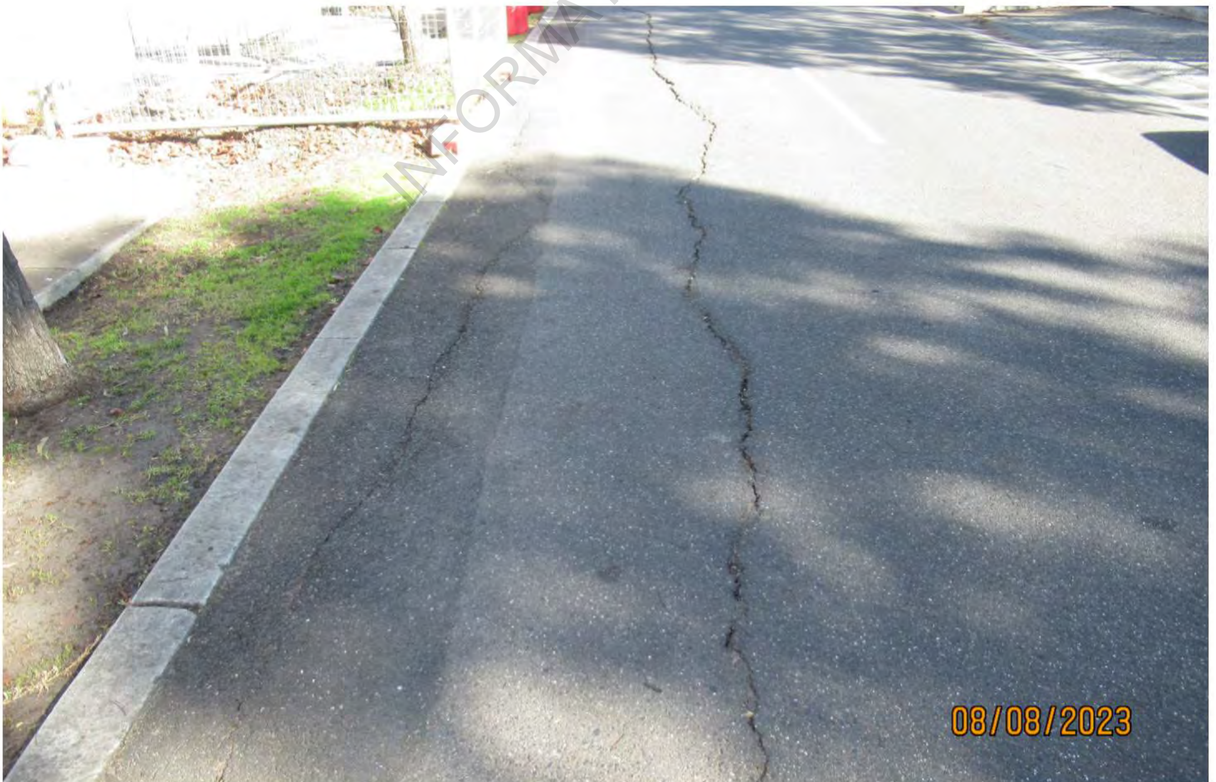
Photo 1.40: Cracking to roadway similar to that observed in April
