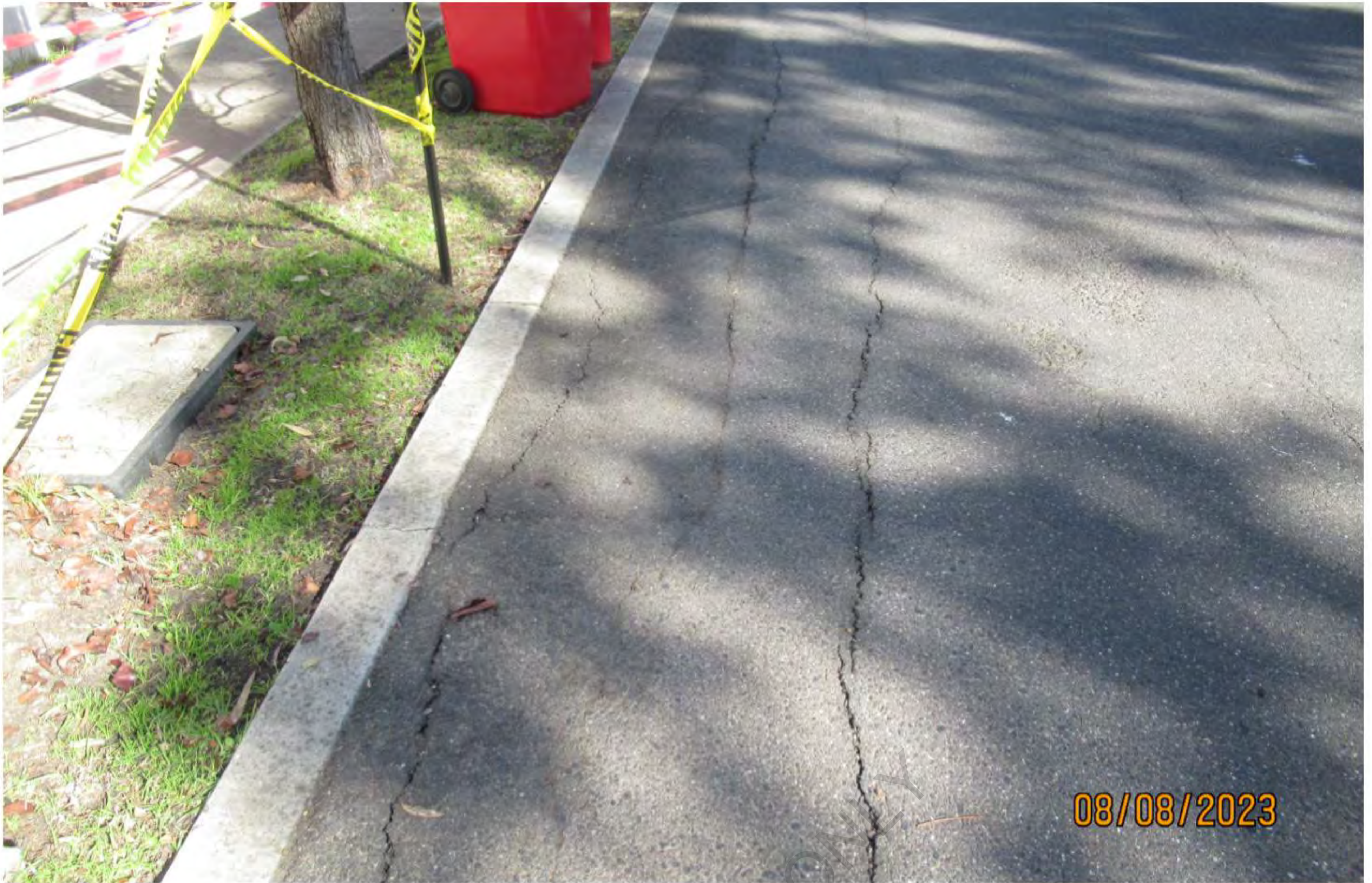
Photo 1.39: Cracking to roadway similar to that observed in April
