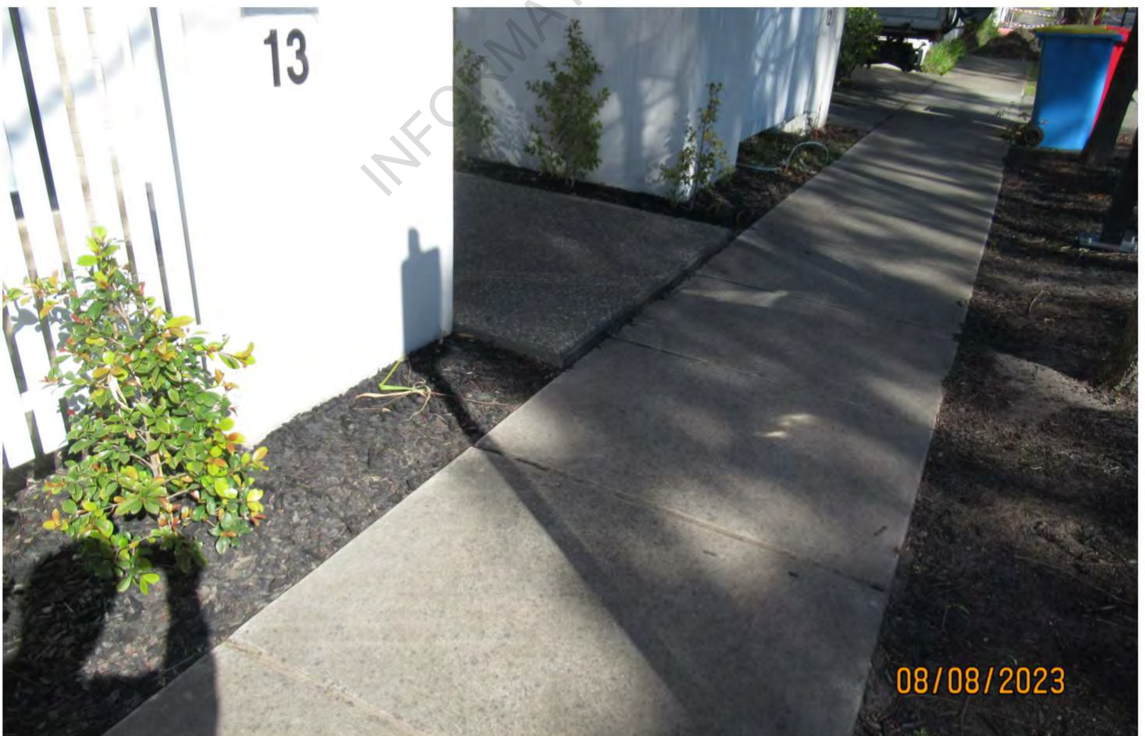
Photo 1.52: Differential settlement between footpath and townhouse pathway
