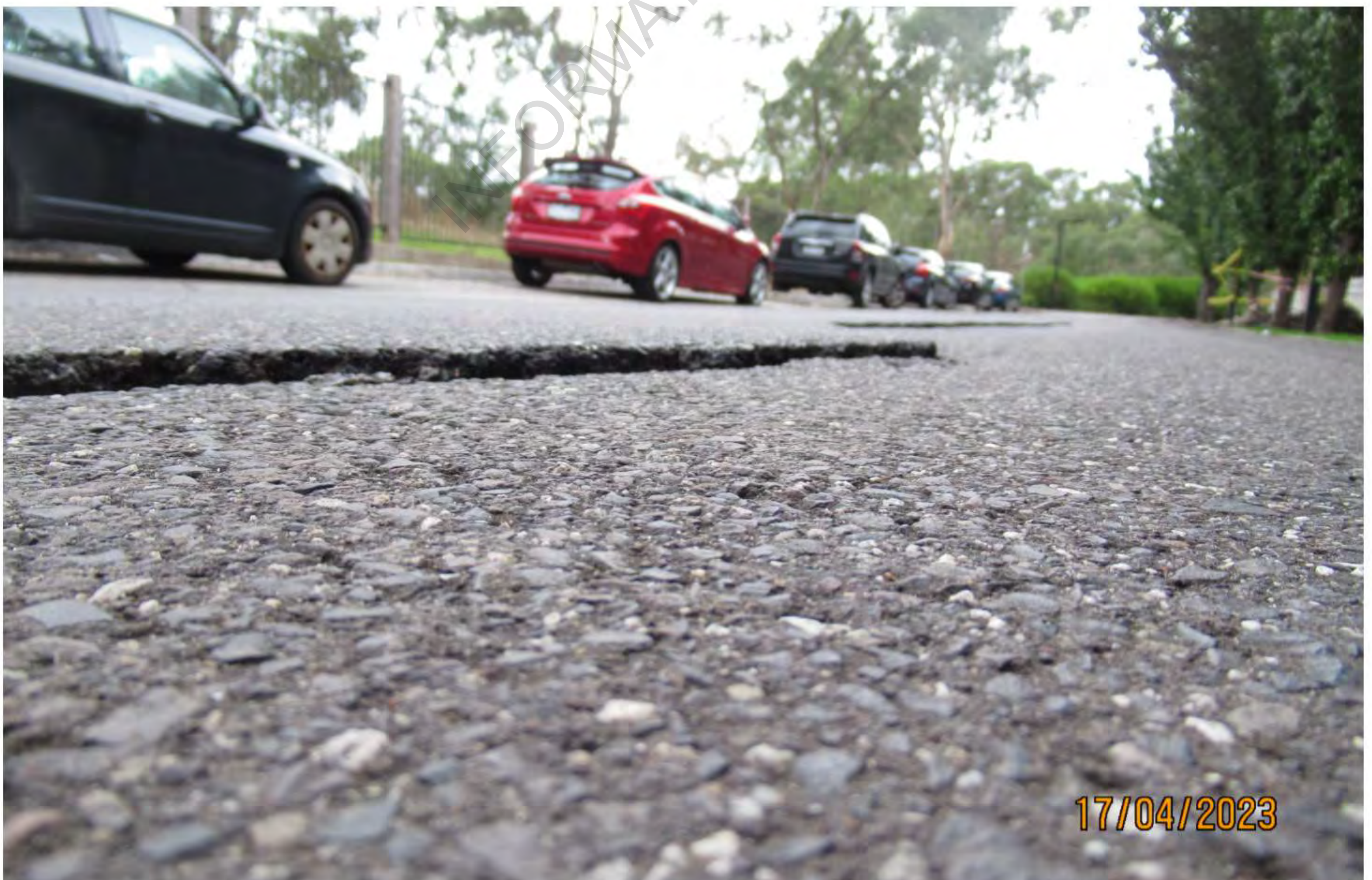
Photo 1.34: Displacement of the road surface across cracks had increased
