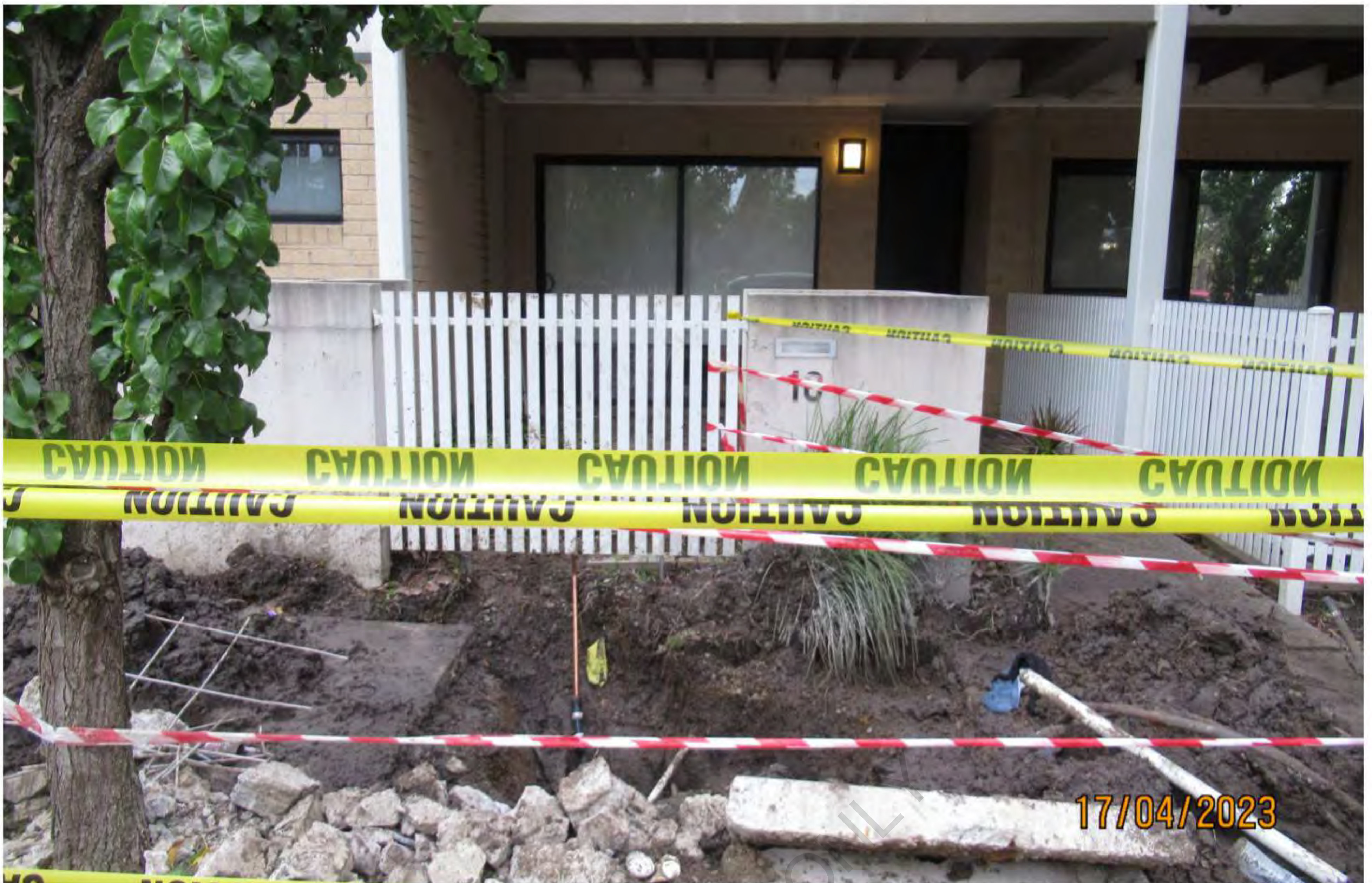
Photo 1.25: Location of water leak in front of 10 Gorman Drive
