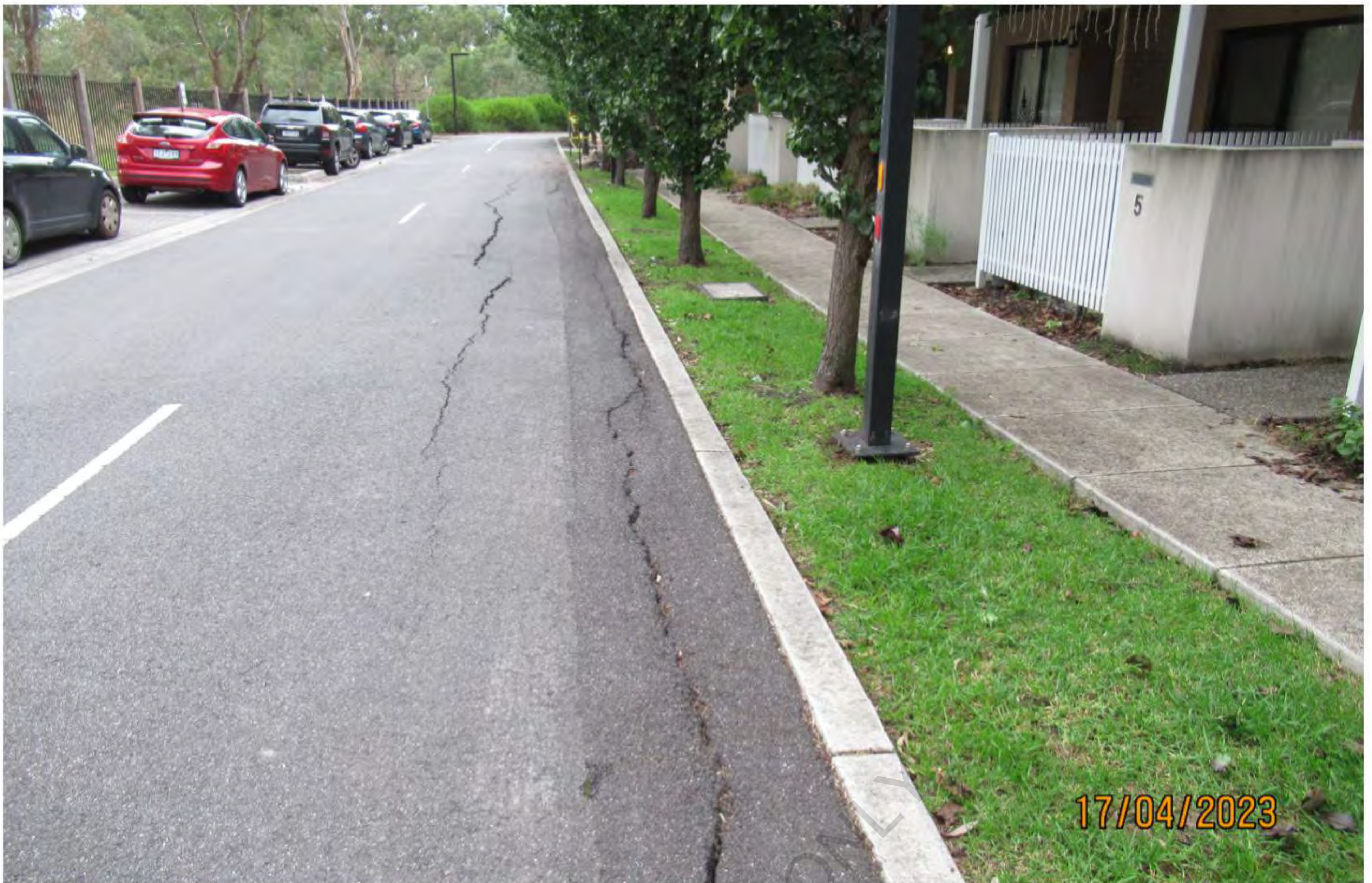
Photo 1.29: Increase in size and extent of longitudinal cracks in roadway
