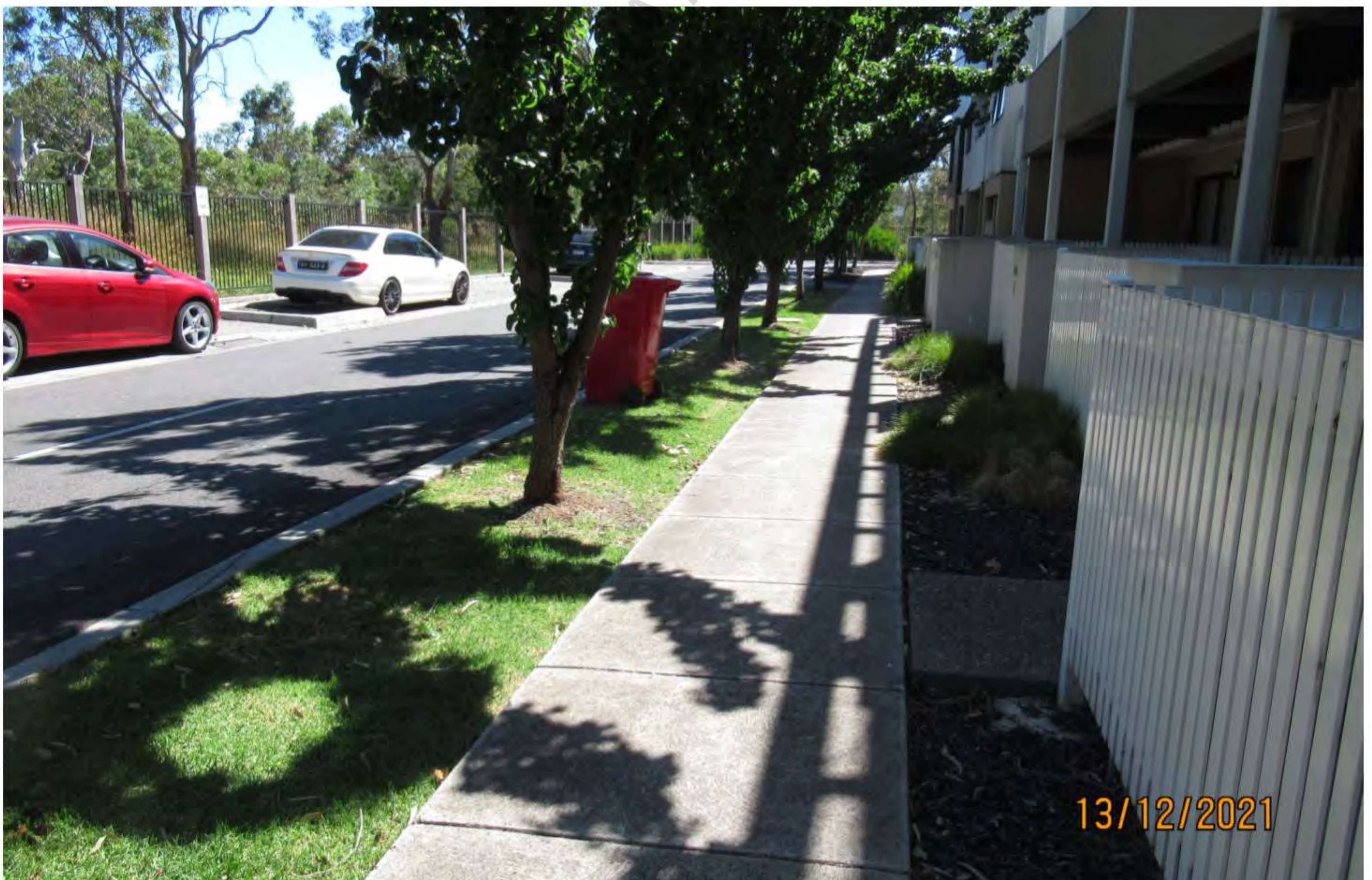
Photo 1.18: Concrete footpath has subsided in various areas
