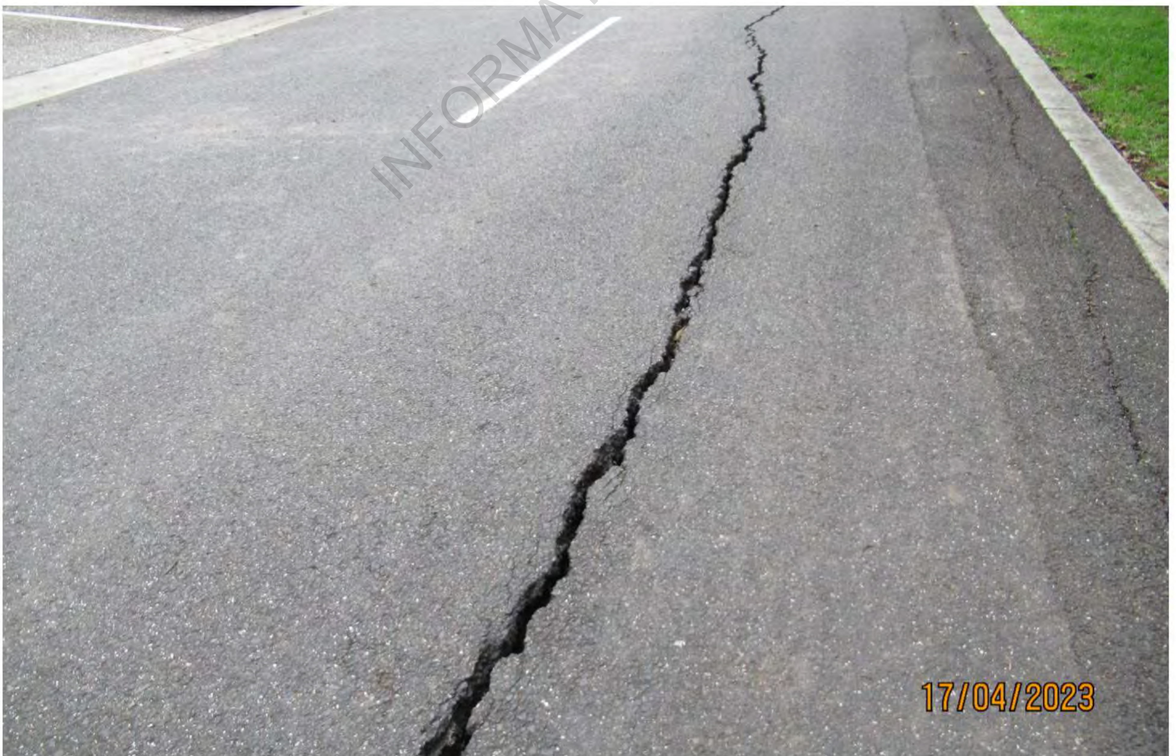
Photo 1.32: Increase in size and extent of longitudinal cracks in roadway
