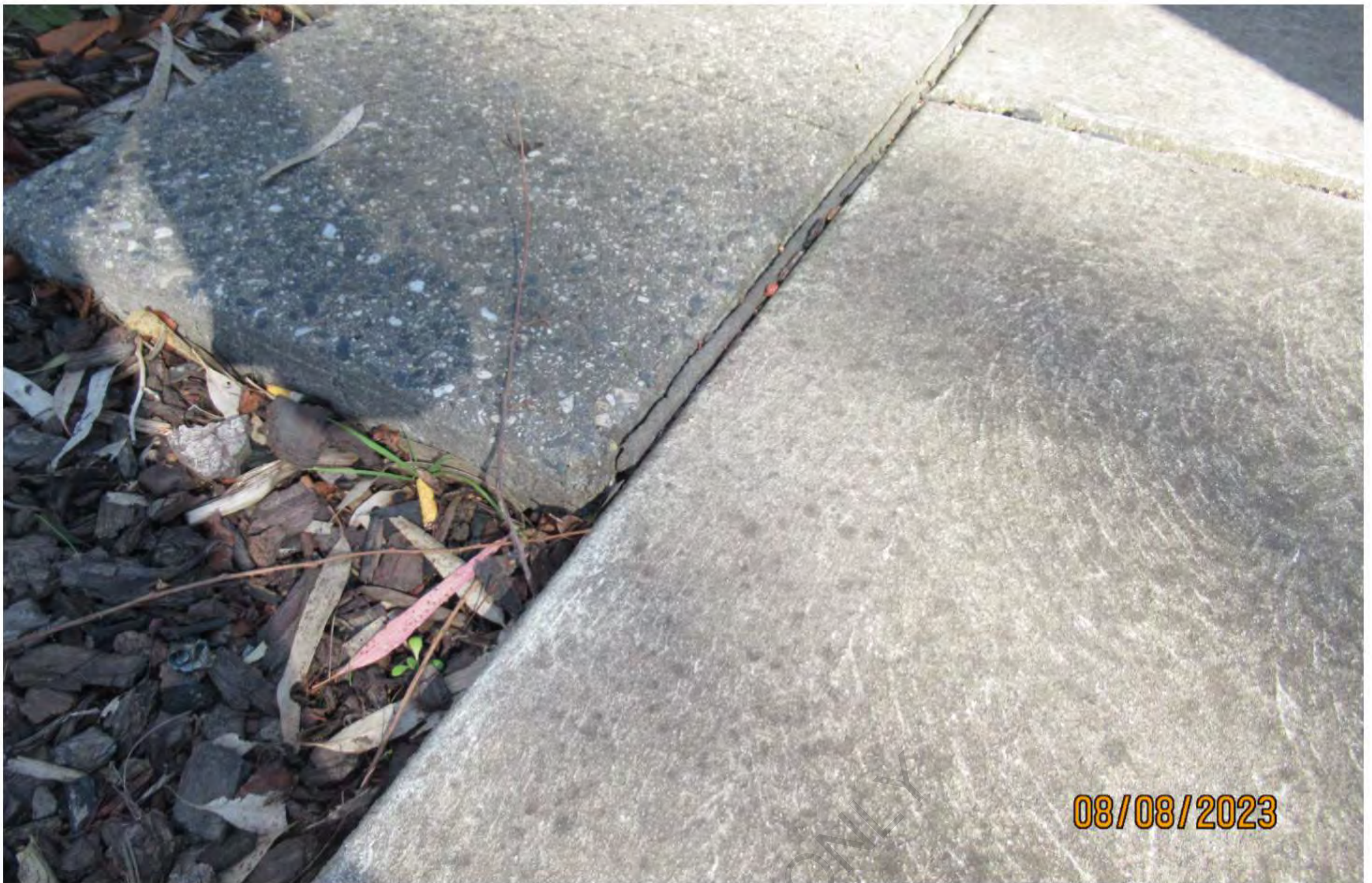
Photo 1.49: Differential settlement between footpath and townhouse pathway
