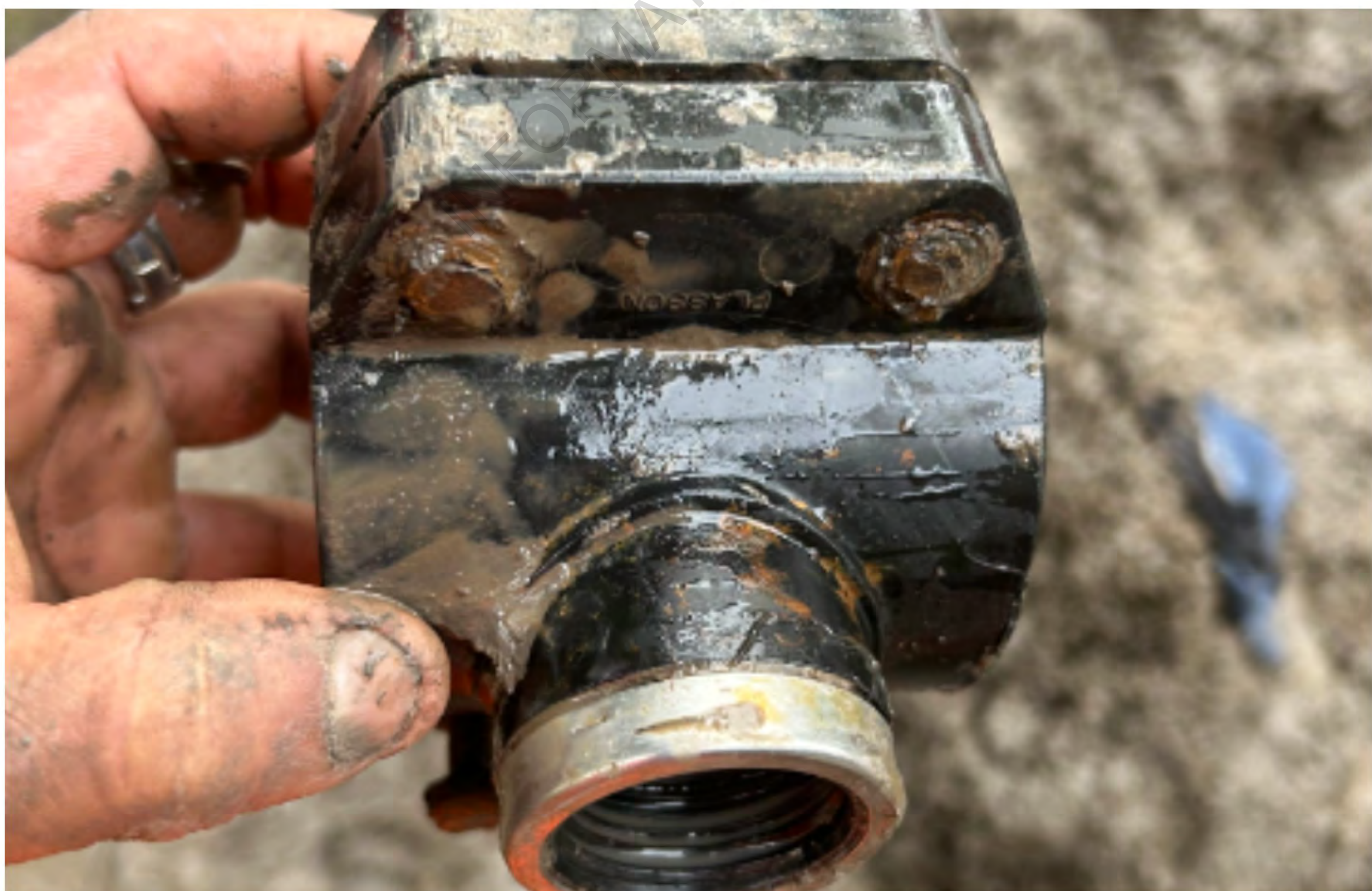
Photo 2.6: Rusted bolts in tapping saddle
