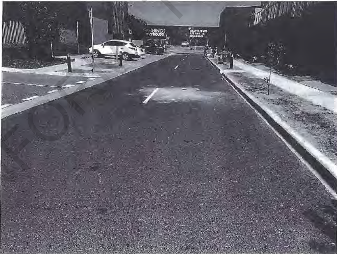
Figure 5-4: Asphalt surface is in good condition (looking west with BH05 in the forefront)
