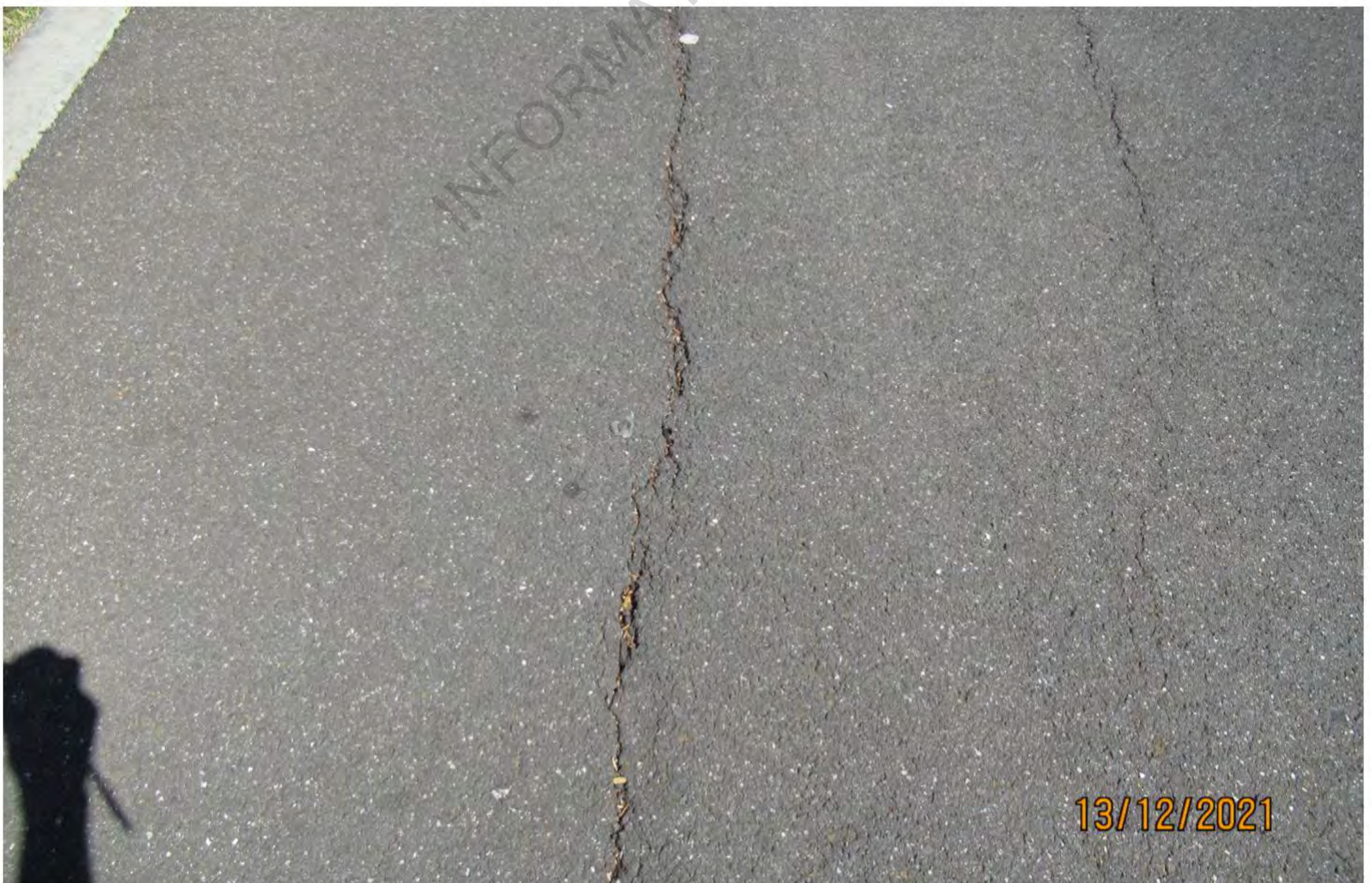
Photo 1.14: Longitudinal cracks in Leg B of Gorman Drive
