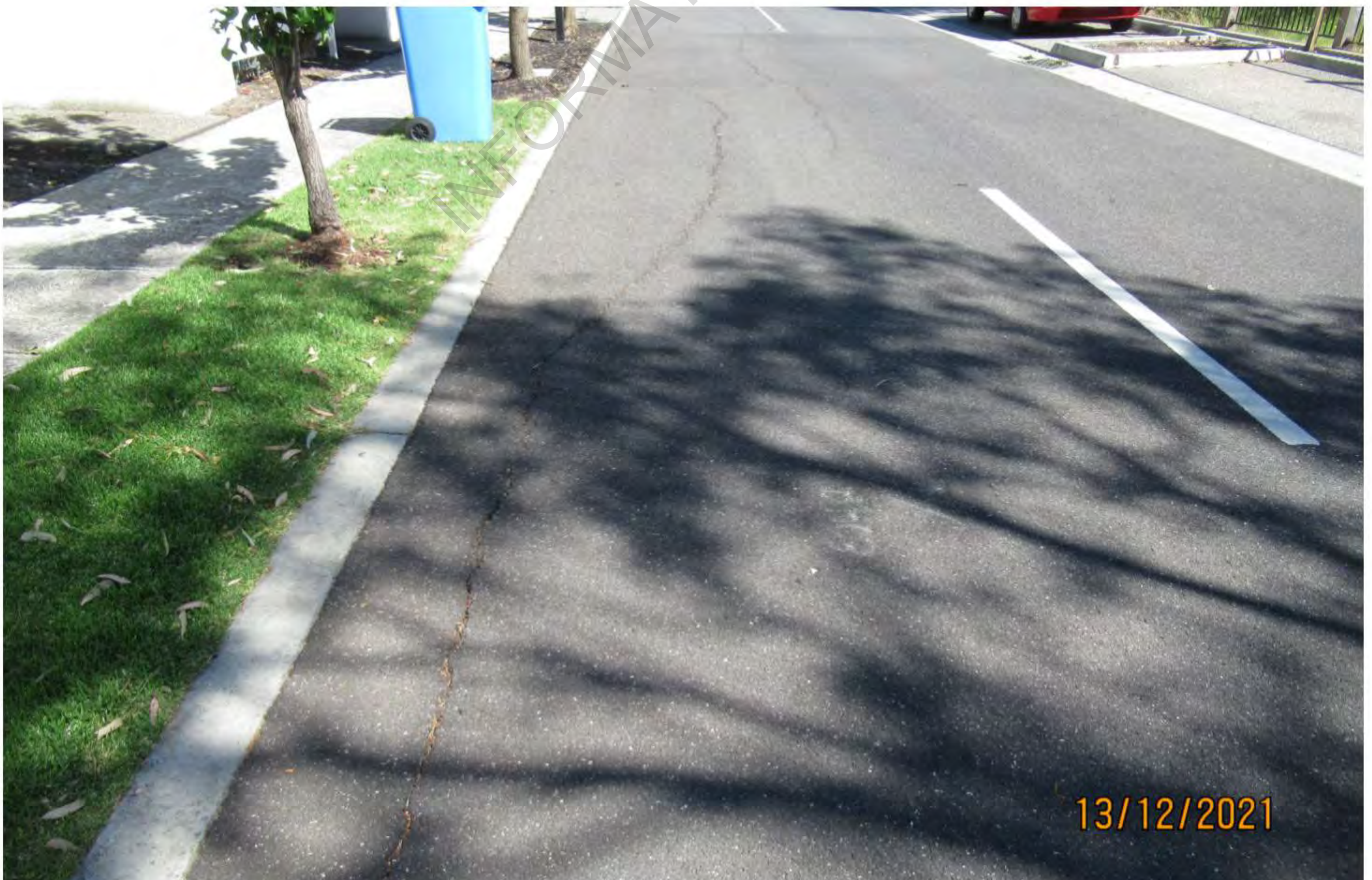
Photo 1.16: Longitudinal cracks in Leg B of Gorman Drive
