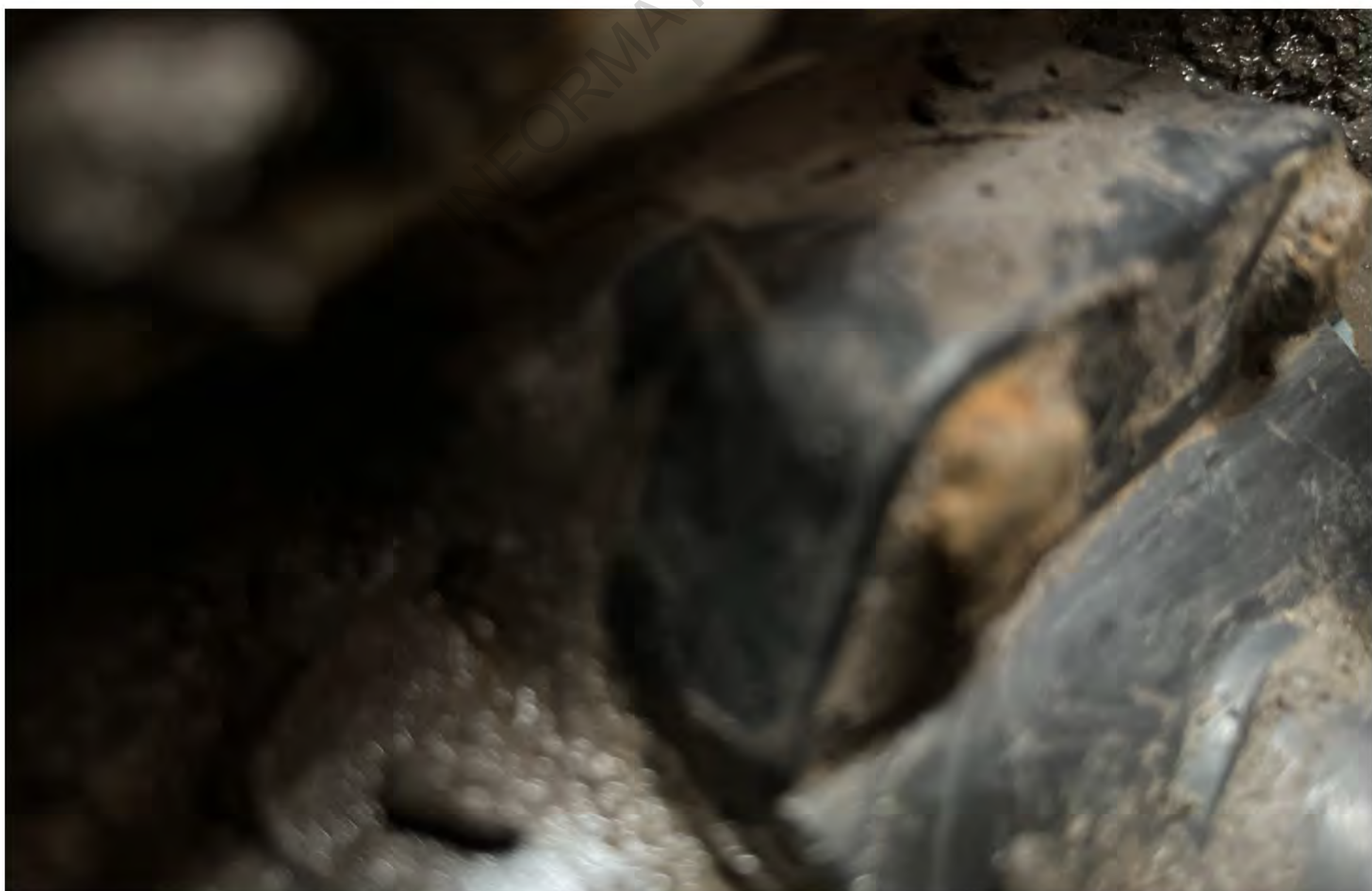
Photo 6: Rusted bolts visible in tapping saddle
