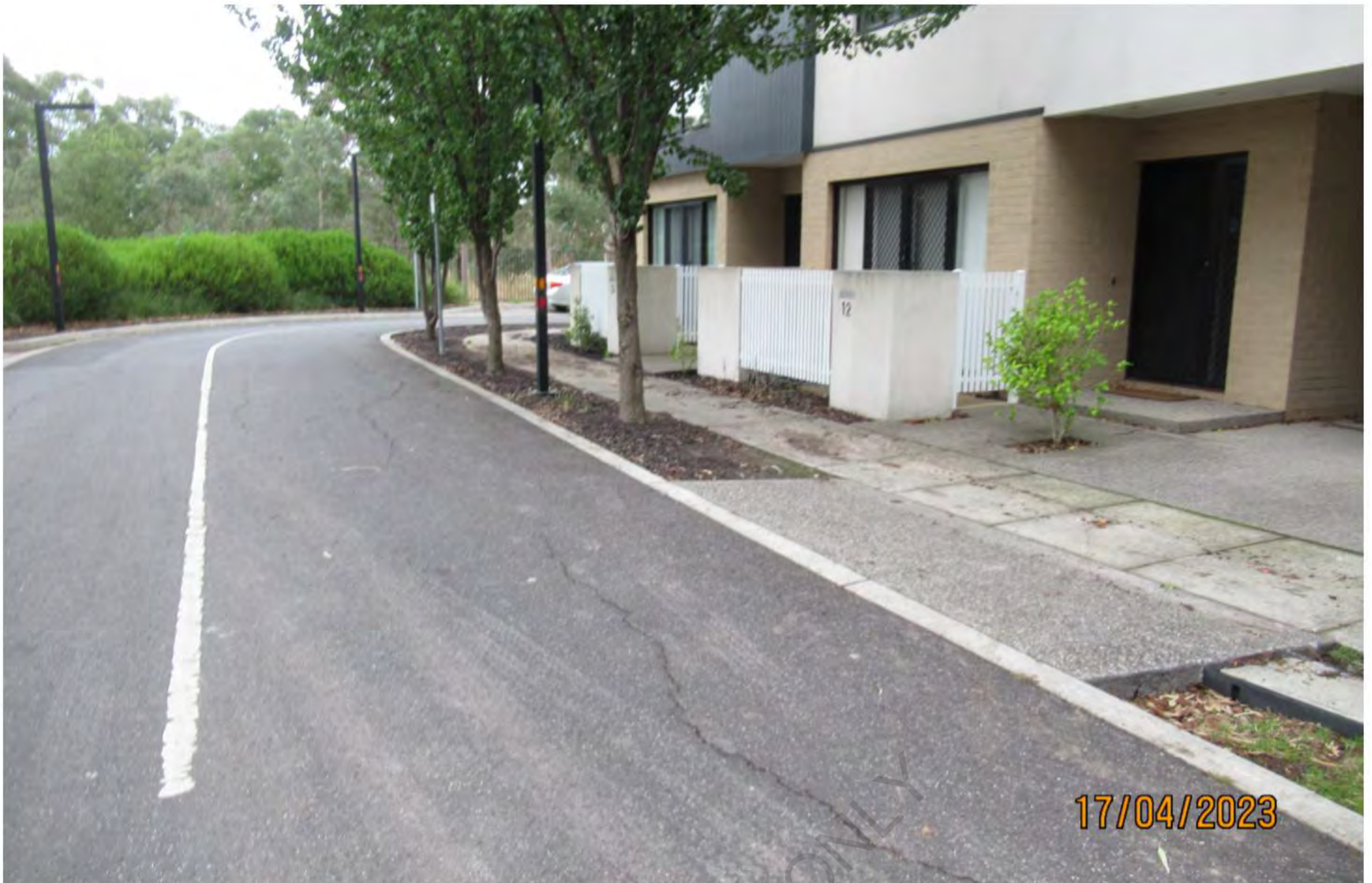
Photo 1.21: Visible signs of water inundation from leak
