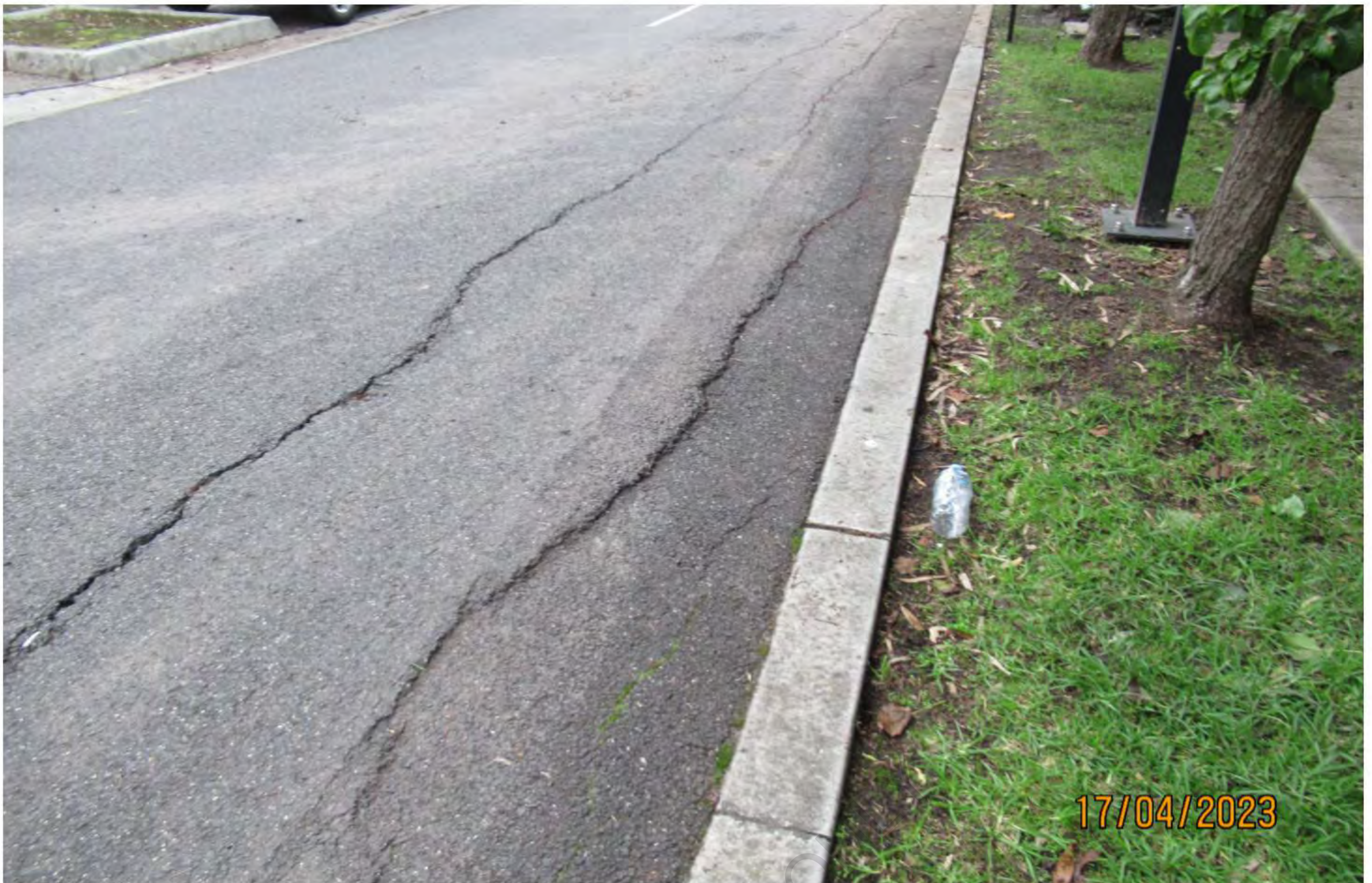
Photo 1.35: Displacement of the road surface across cracks had increased
