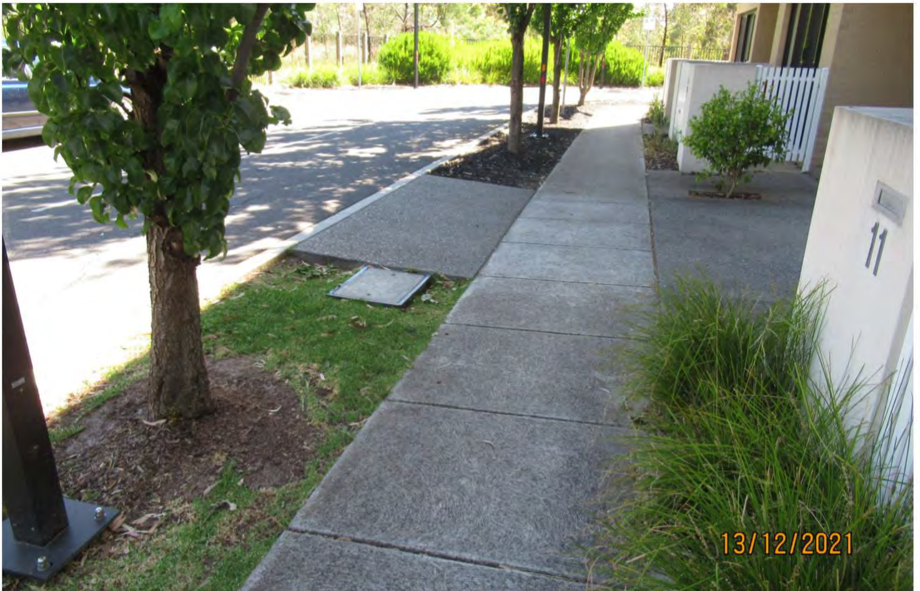
Photo 1.19: Concrete footpath has subsided in various areas
