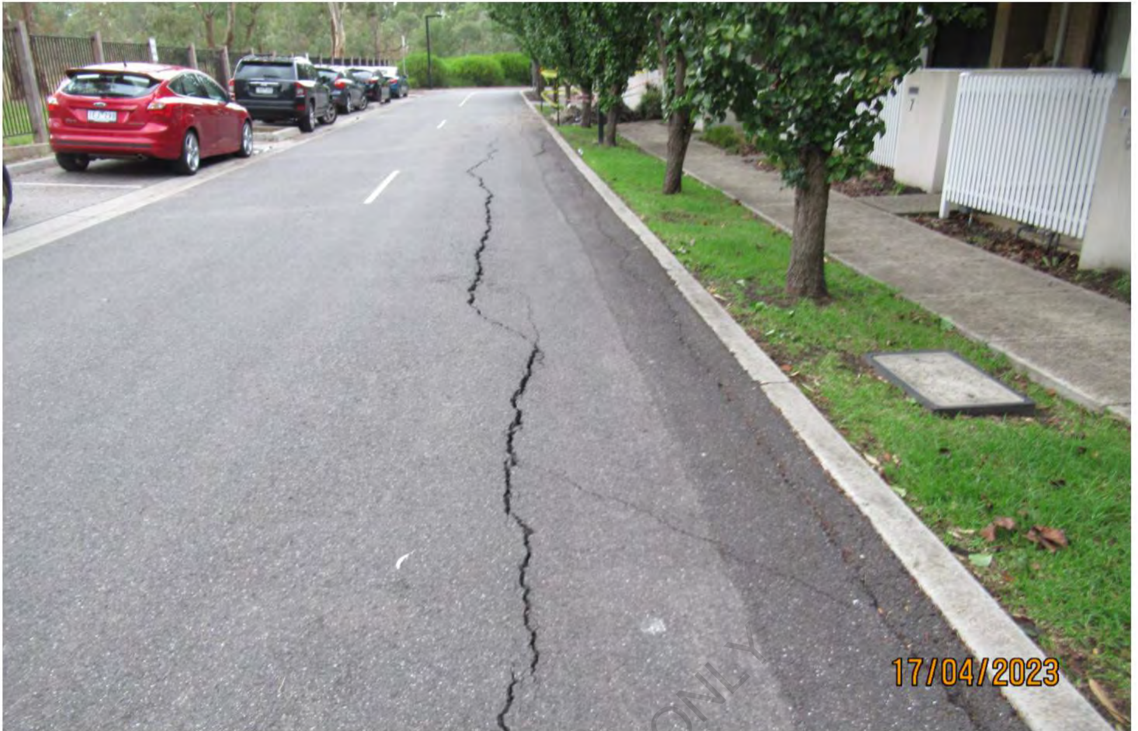
Photo 1.33: Displacement of the road surface across cracks had increased
