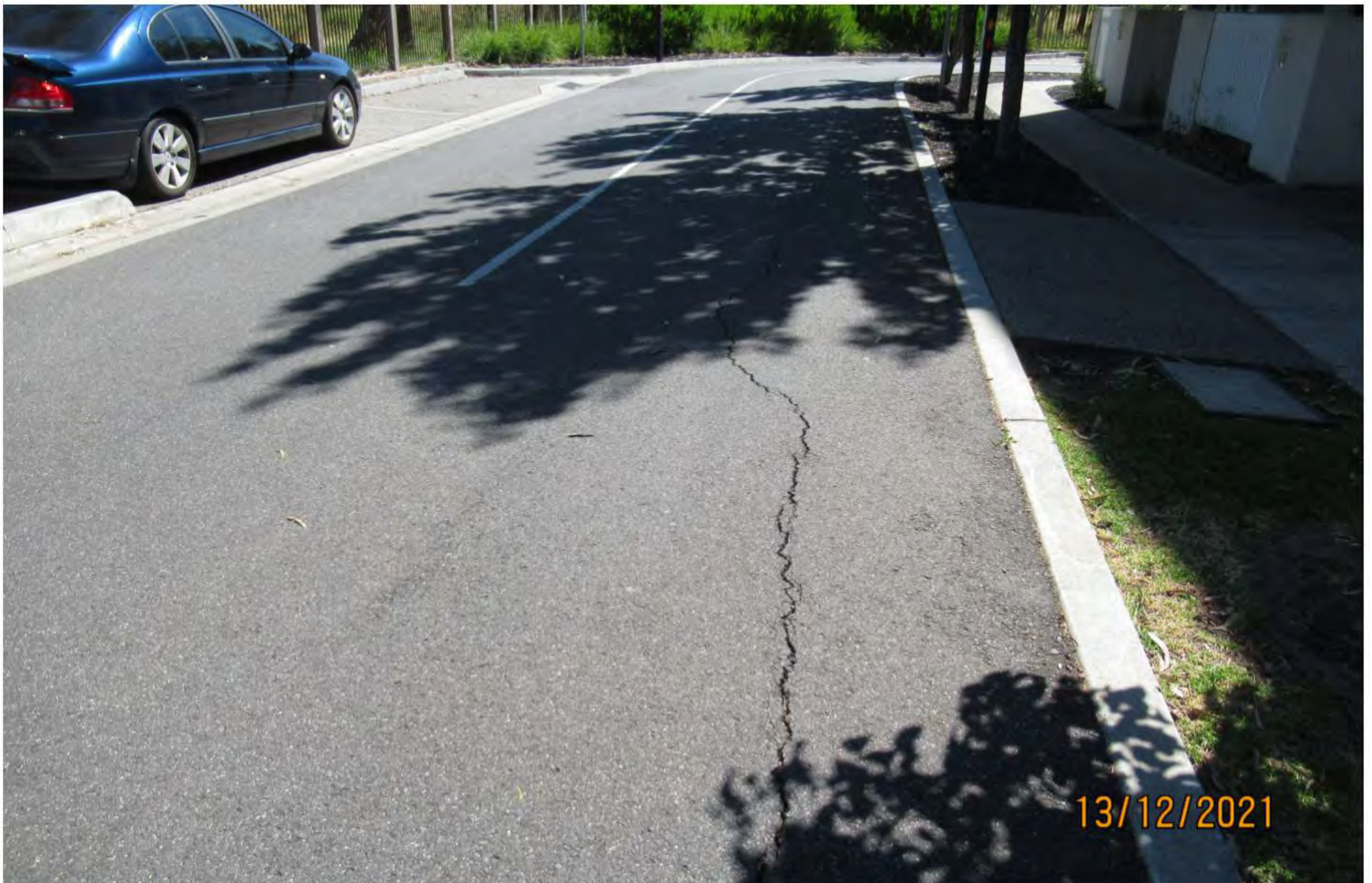
Photo 1.11: Longitudinal cracks in Leg A of Gorman Drive
