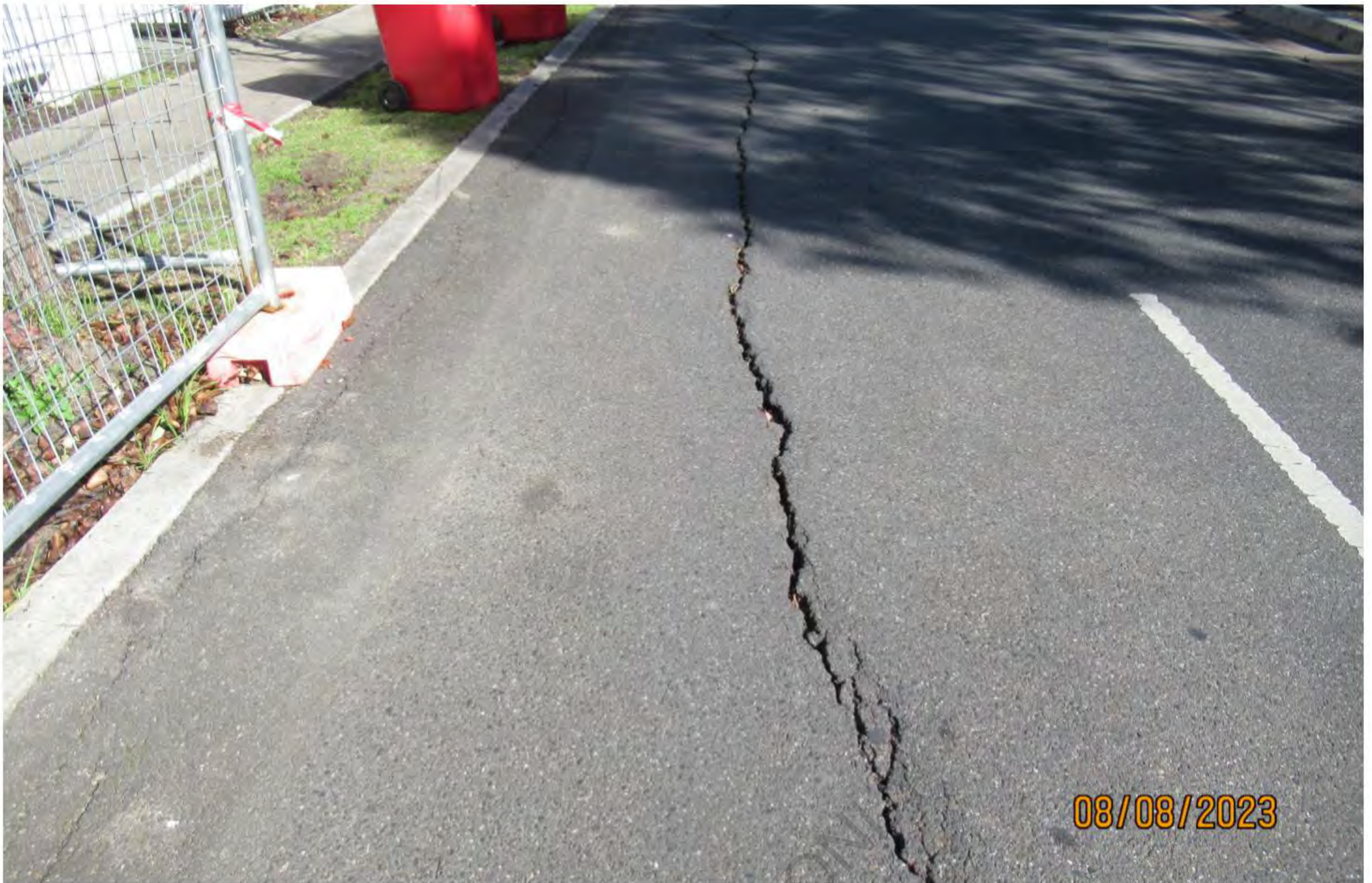
Photo 1.41: Cracking to roadway similar to that observed in April
