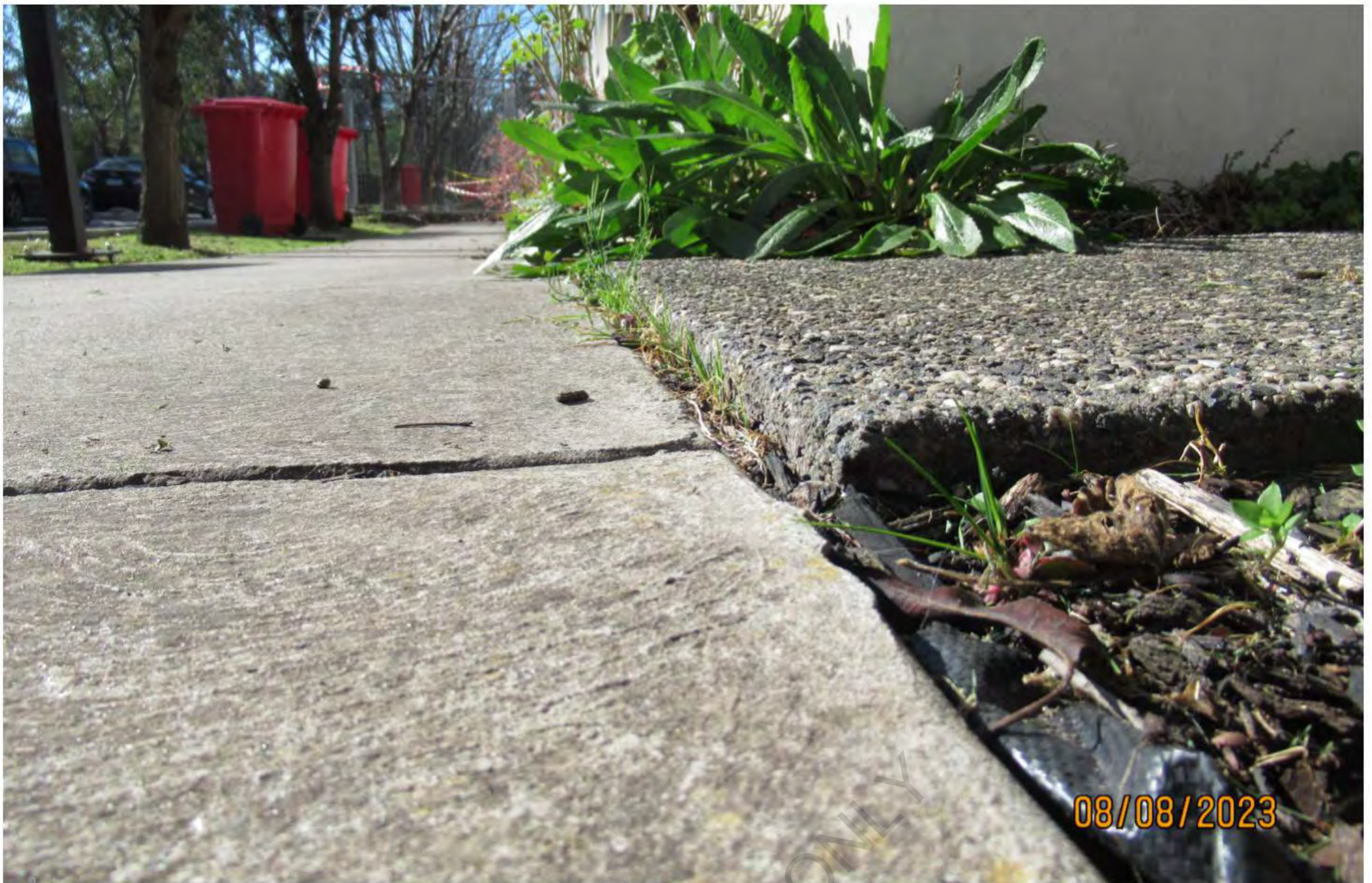
Photo 1.47: Differential settlement between footpath and townhouse pathway
