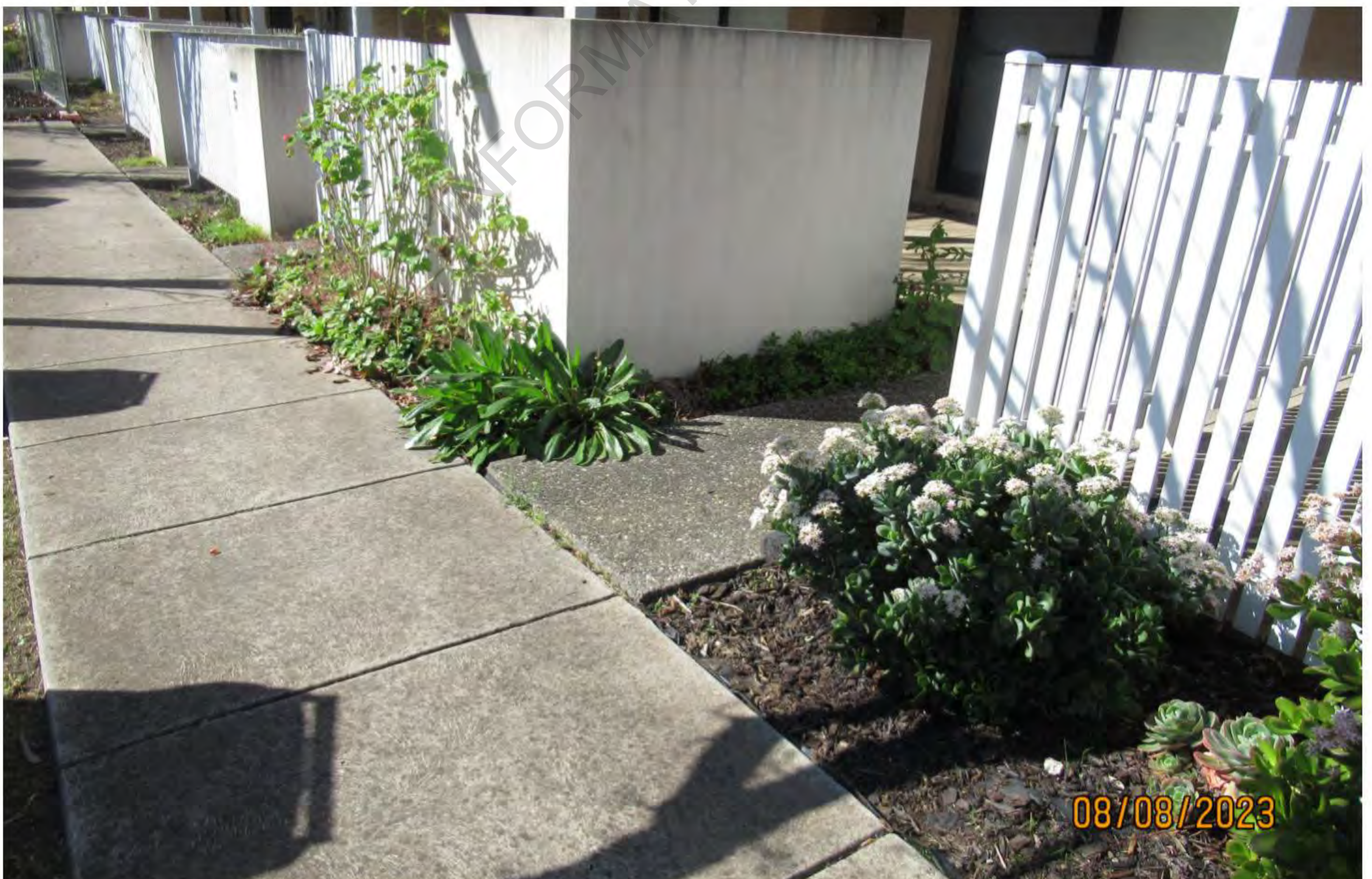
Photo 1.46: Differential settlement between footpath and townhouse pathway
