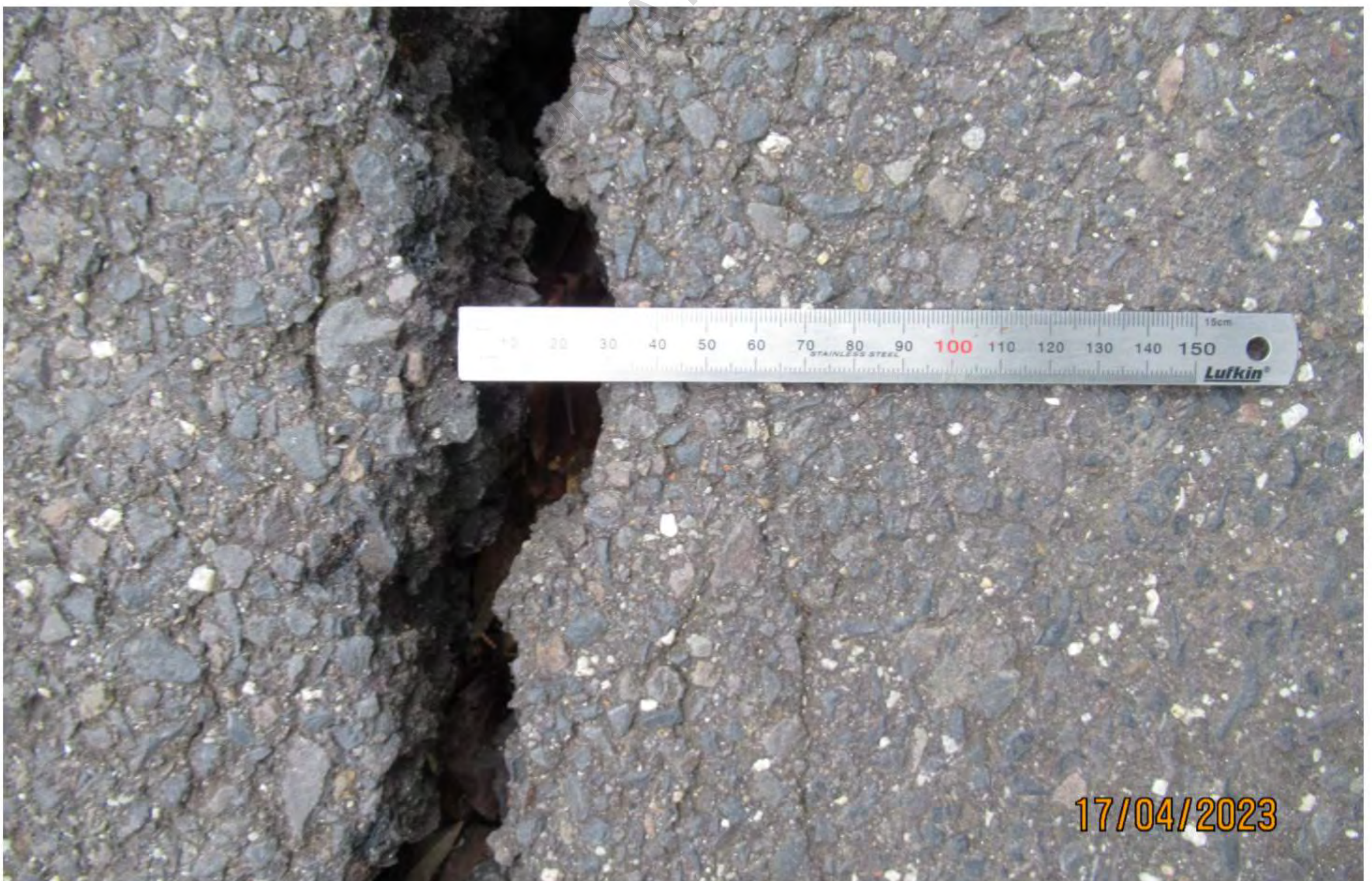
Photo 1.38: Measurement of crack width
