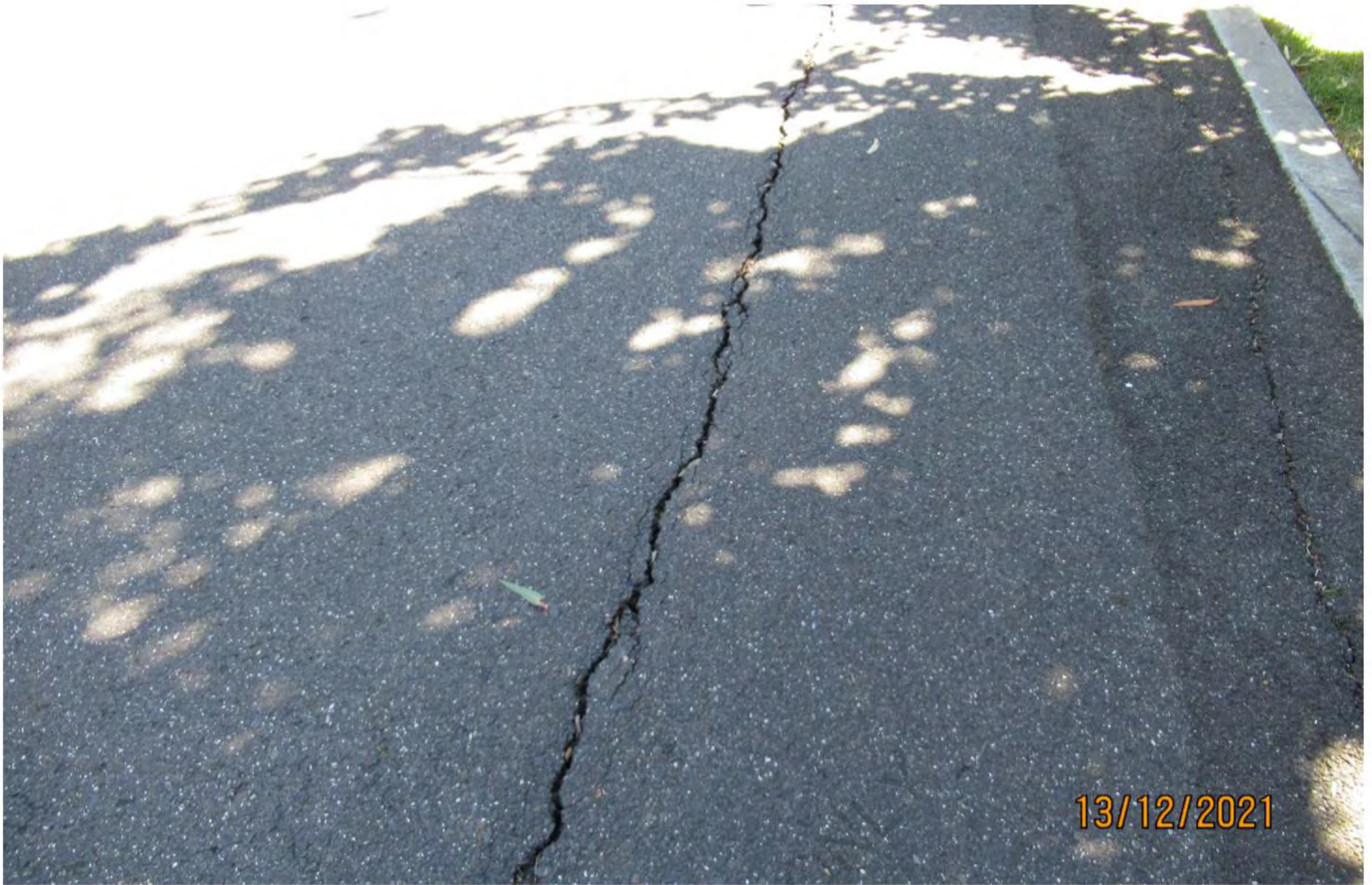
Photo 1.9: Longitudinal cracks in Leg A of Gorman Drive
