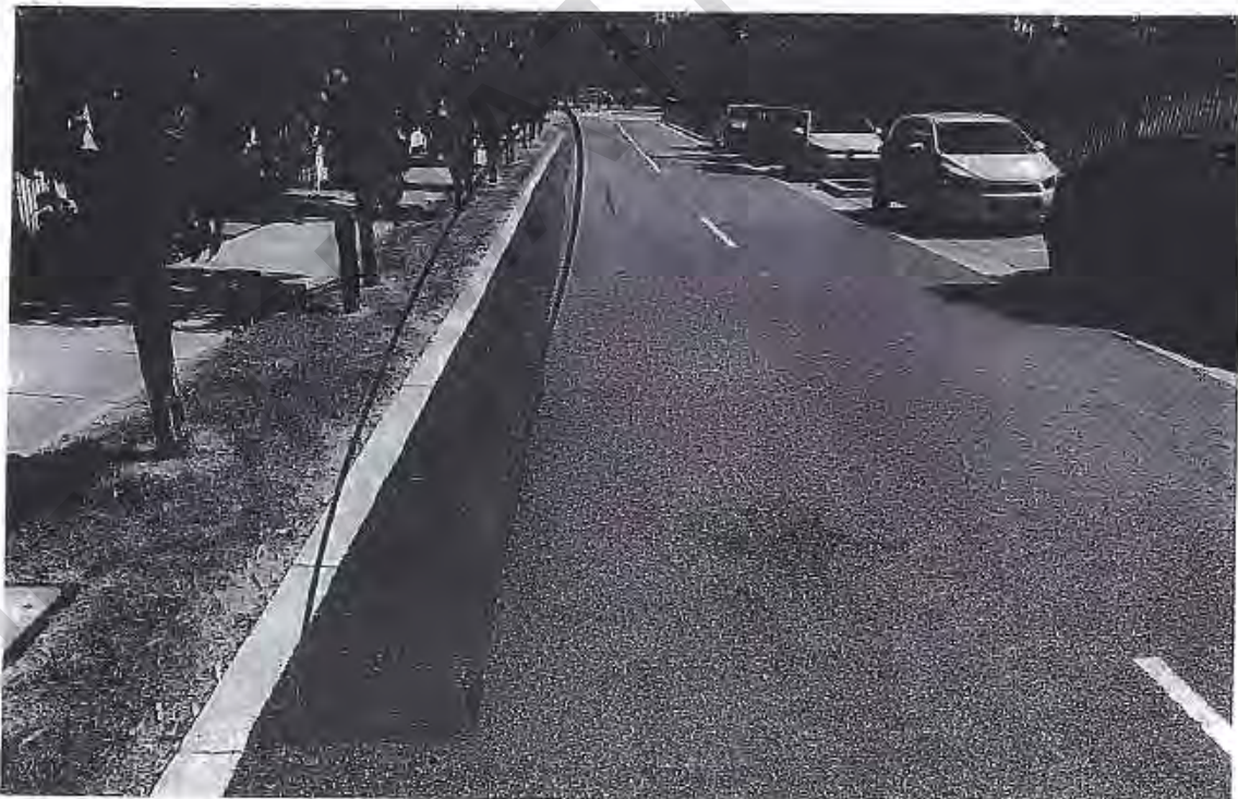
Figure 5-2: Longitudinal cracks in the west bound lane within a recent reinstated pavement patching.
