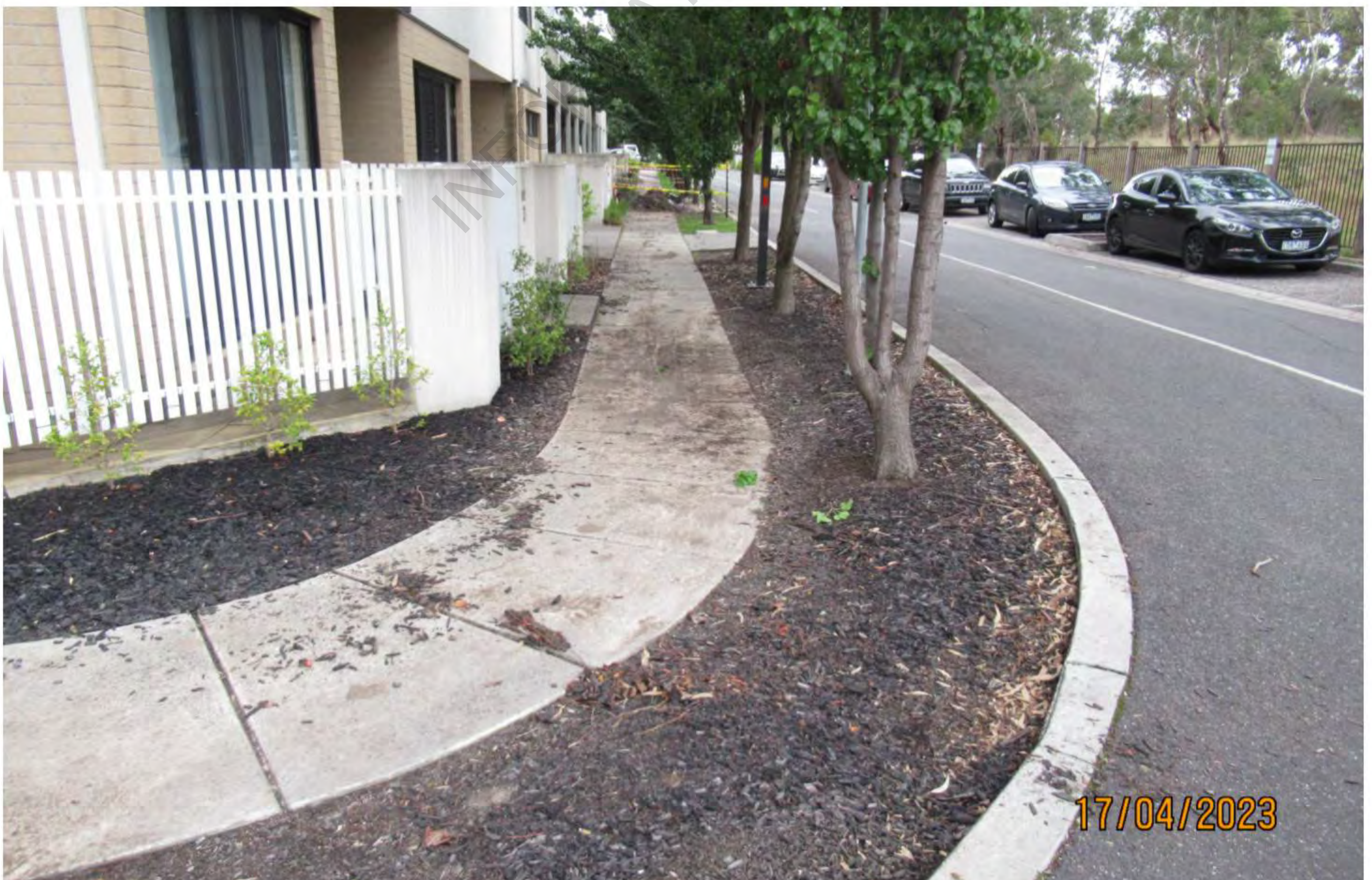
Photo 1.22: Visible signs of water inundation from lea
