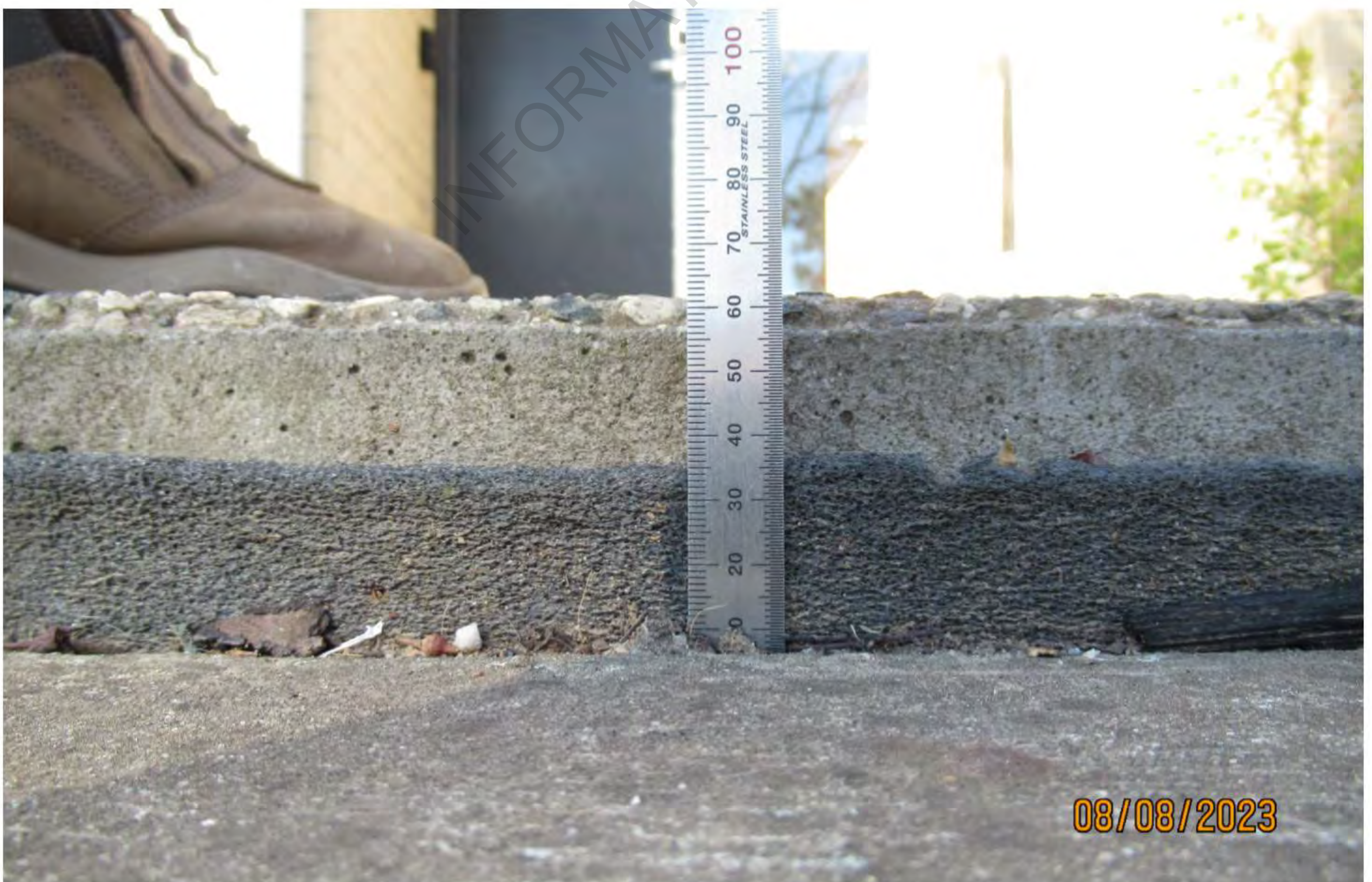
Photo 1.54: Differential settlement between footpath and townhouse pathway
