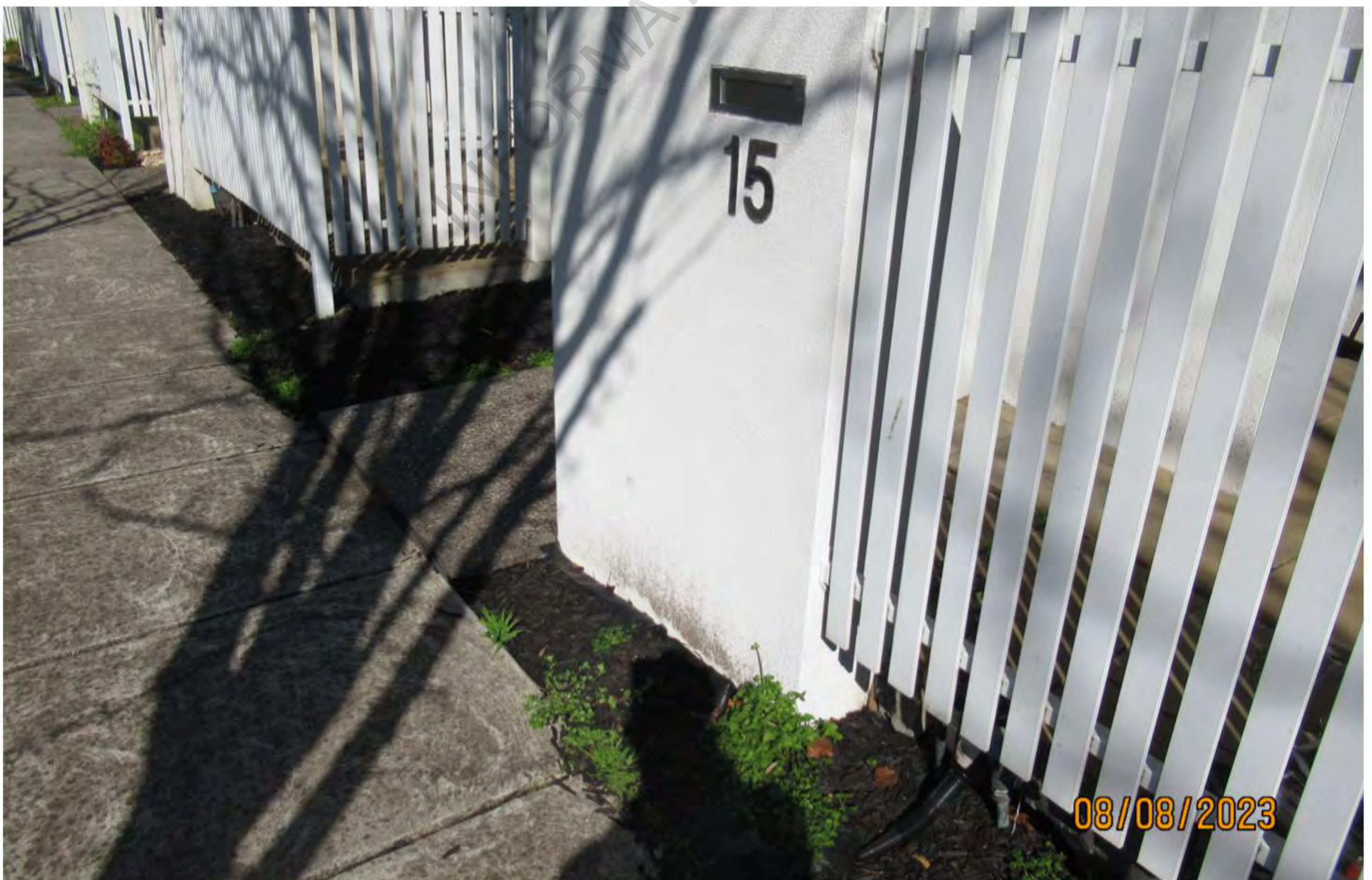
Photo 1.50: Differential settlement between footpath and townhouse pathway
