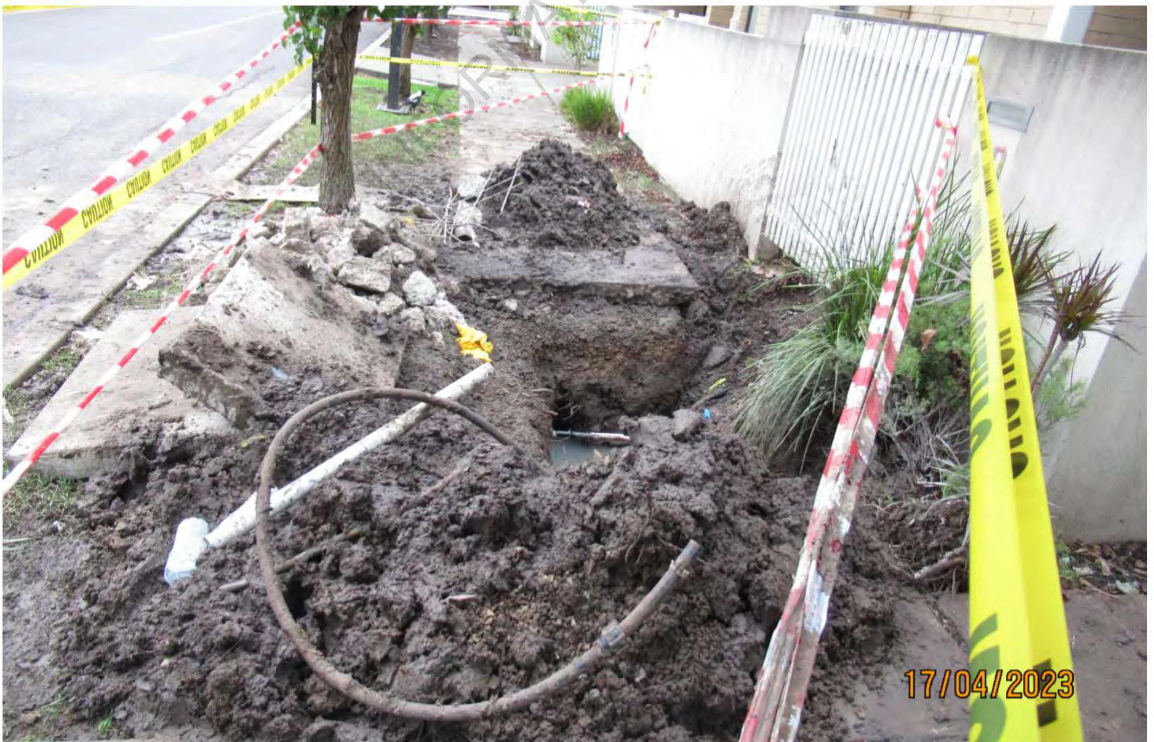
Photo 1.26: Location of water leak in front of 10 Gorman Drive
