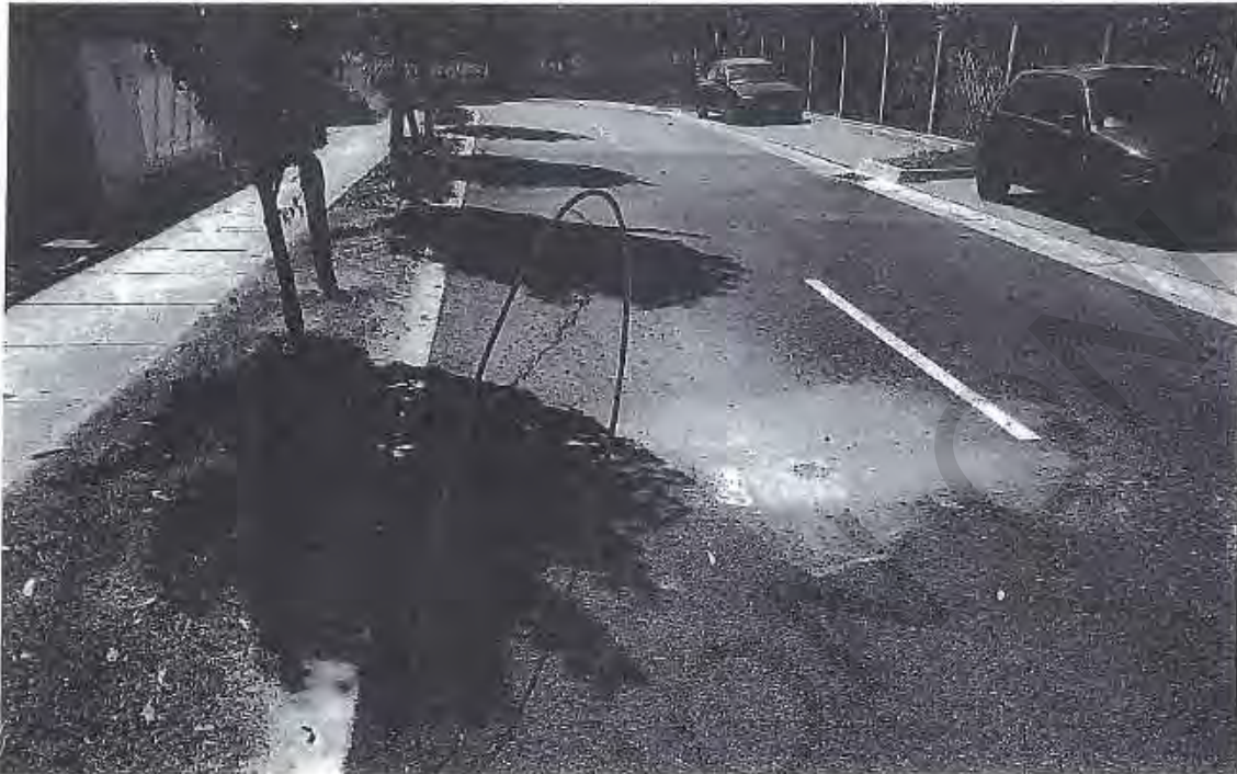
Figure 5-3: Longitudinal cracks in the west bound lane within a newly sealed or repaired section.
