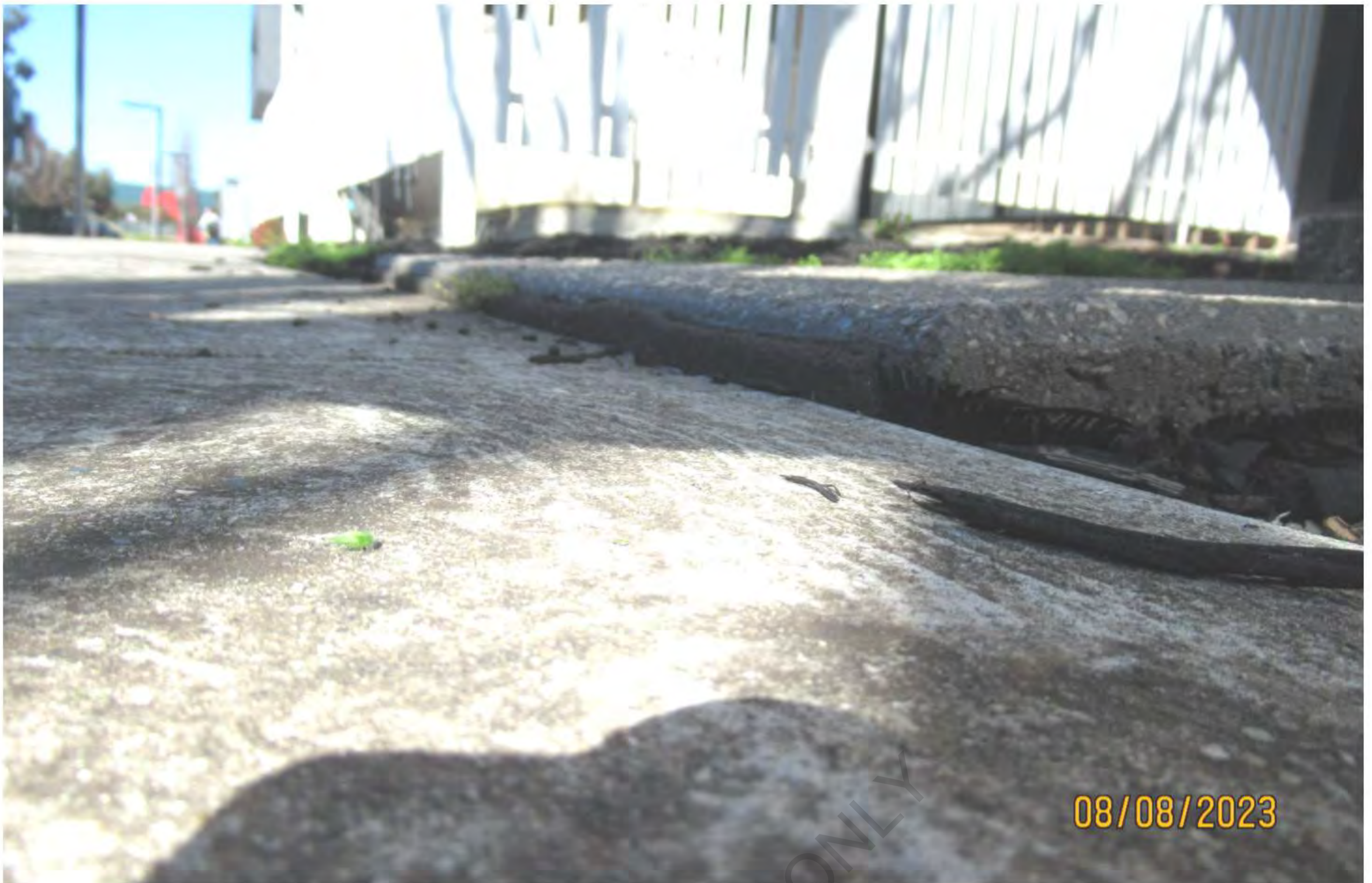
Photo 1.51: Differential settlement between footpath and townhouse pathway
