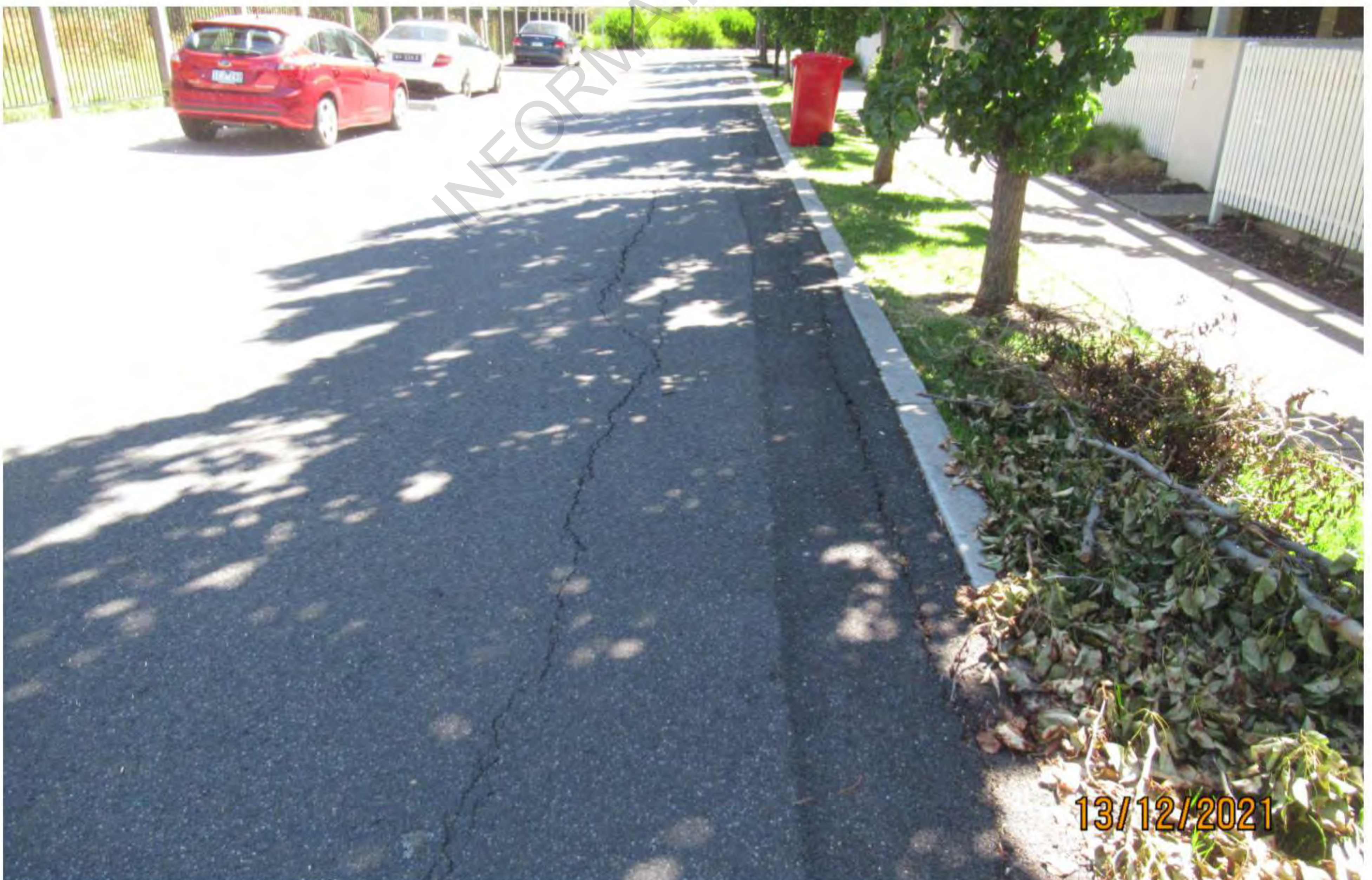
Photo 1.8: Longitudinal cracks in Leg A of Gorman Drive
