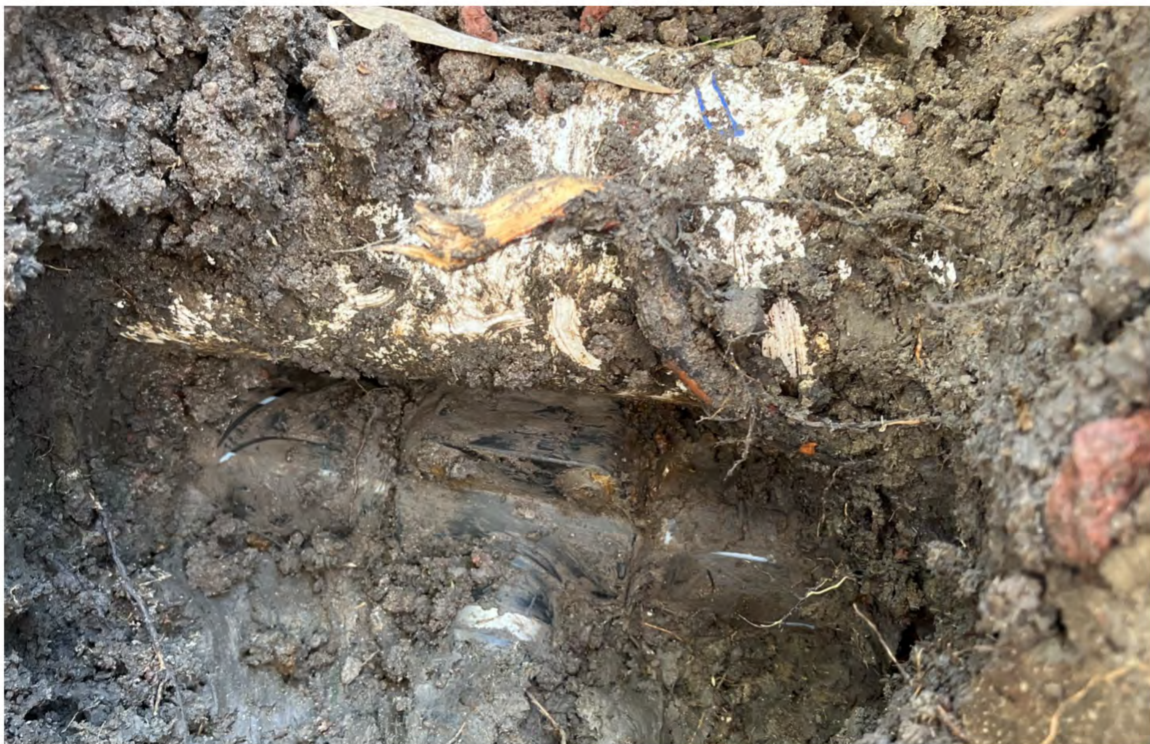
Photo 5: Rusted bolts visible in tapping saddle at water connection
