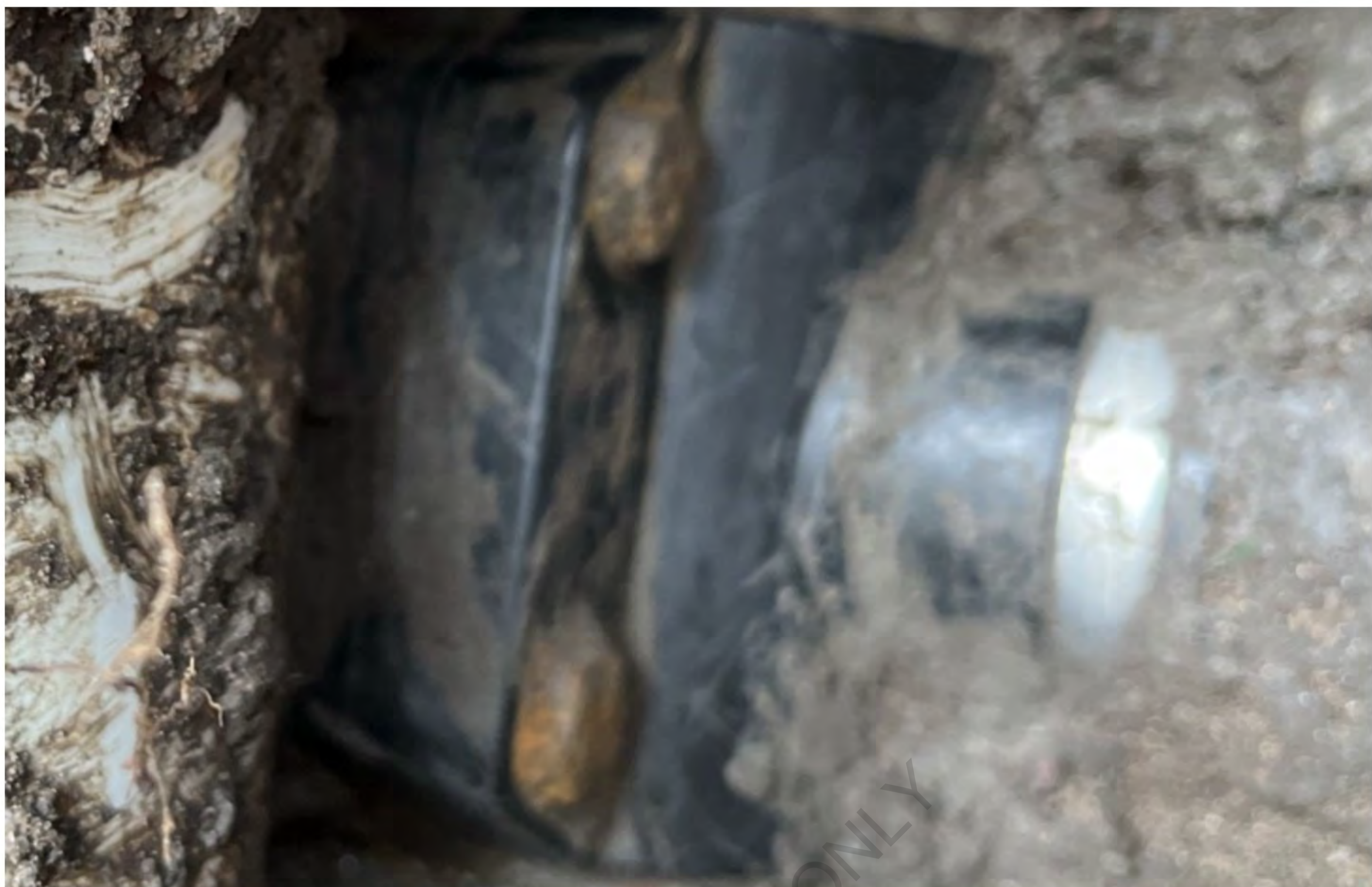
Photo 2.5: Rusted bolts in tapping saddle uncovered
