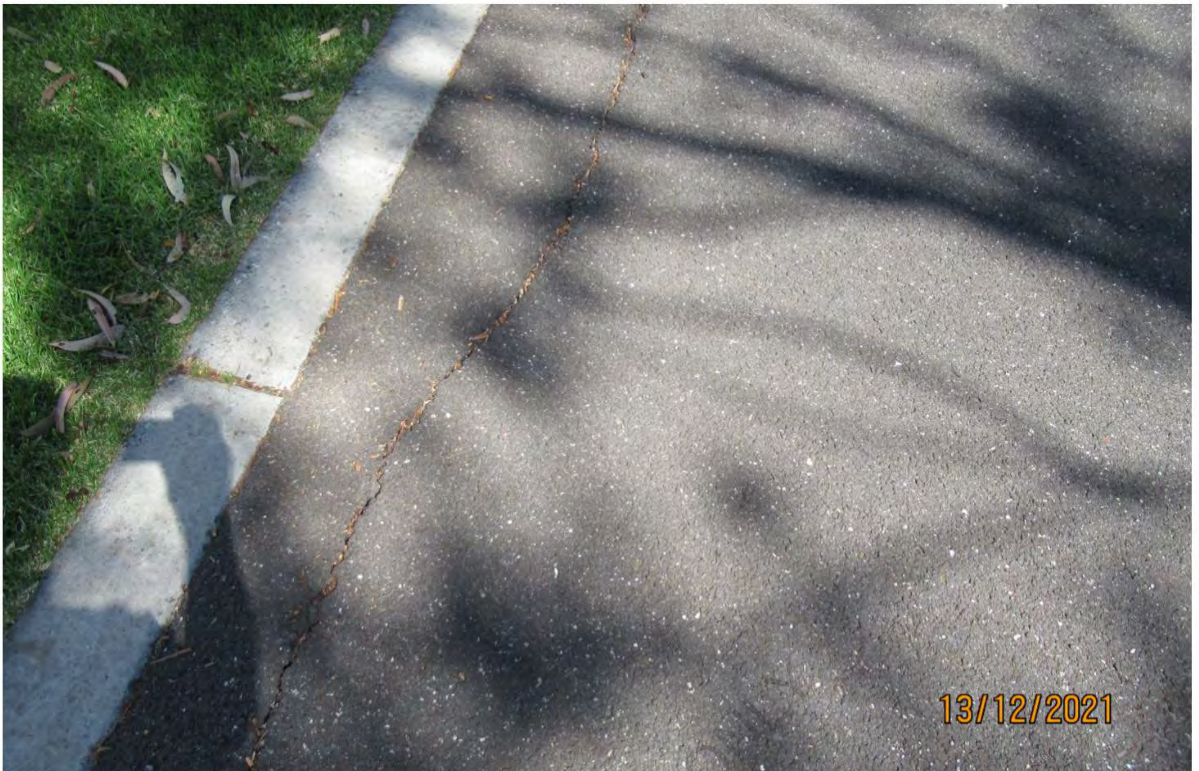
Photo 1.15: Longitudinal cracks in Leg B of Gorman Drive
