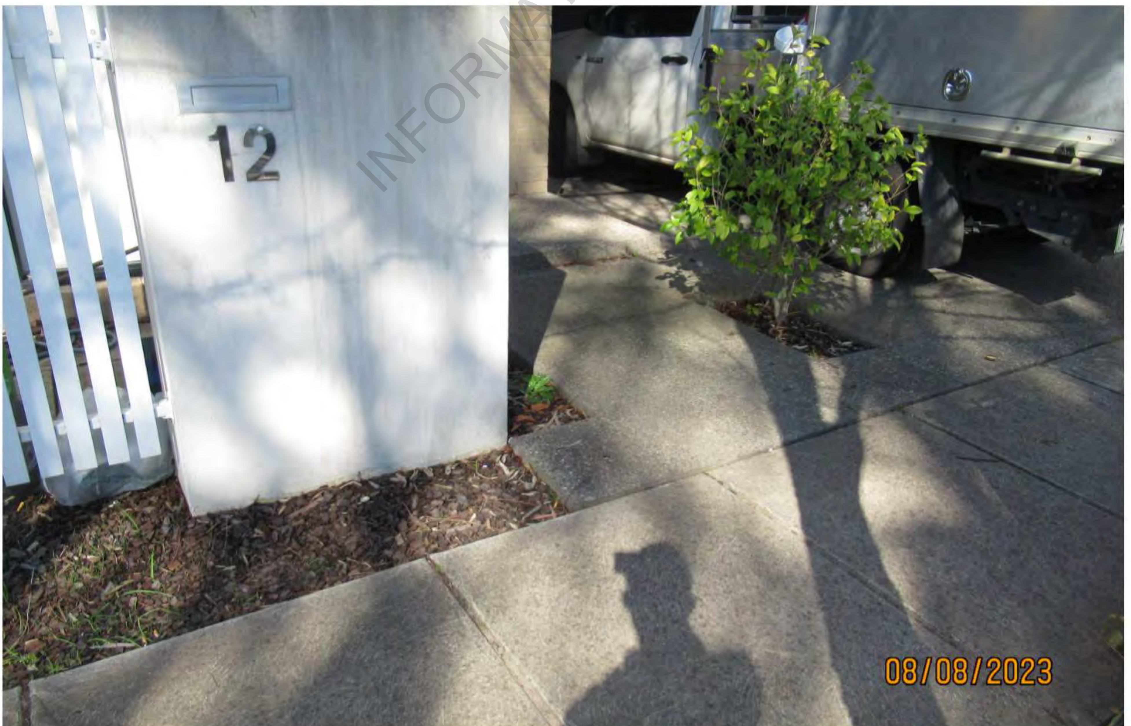
Photo 1.48: Differential settlement between footpath and townhouse pathway
