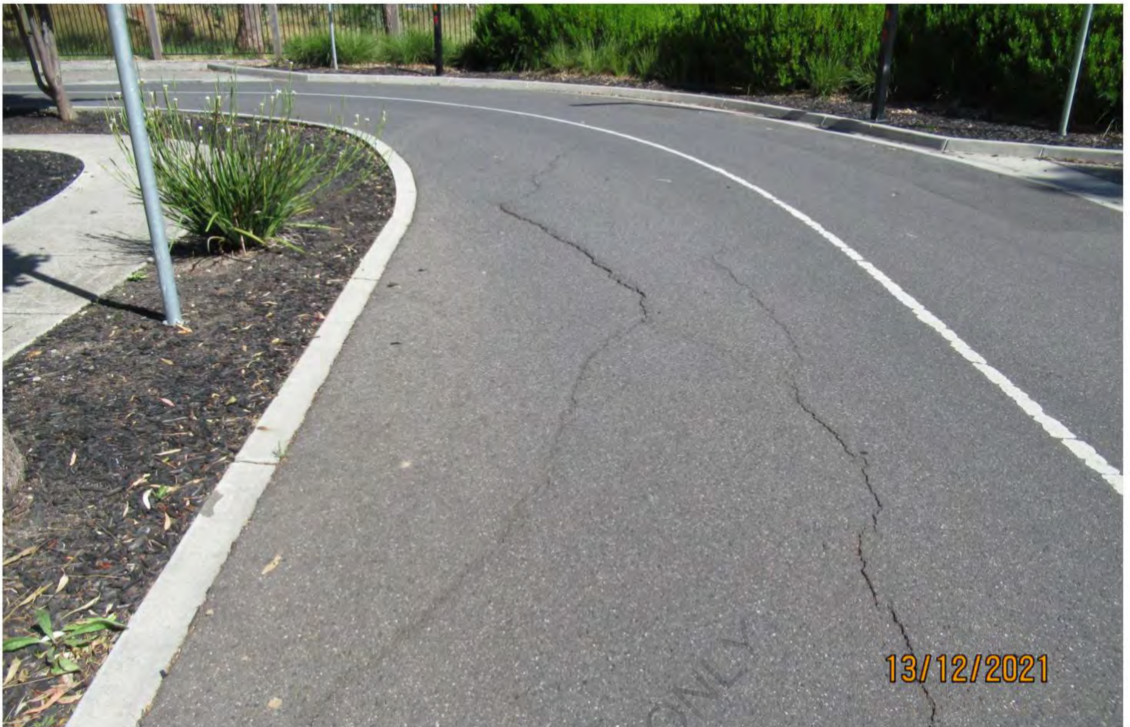
Photo 1.13: Longitudinal cracks in Leg B of Gorman Drive
