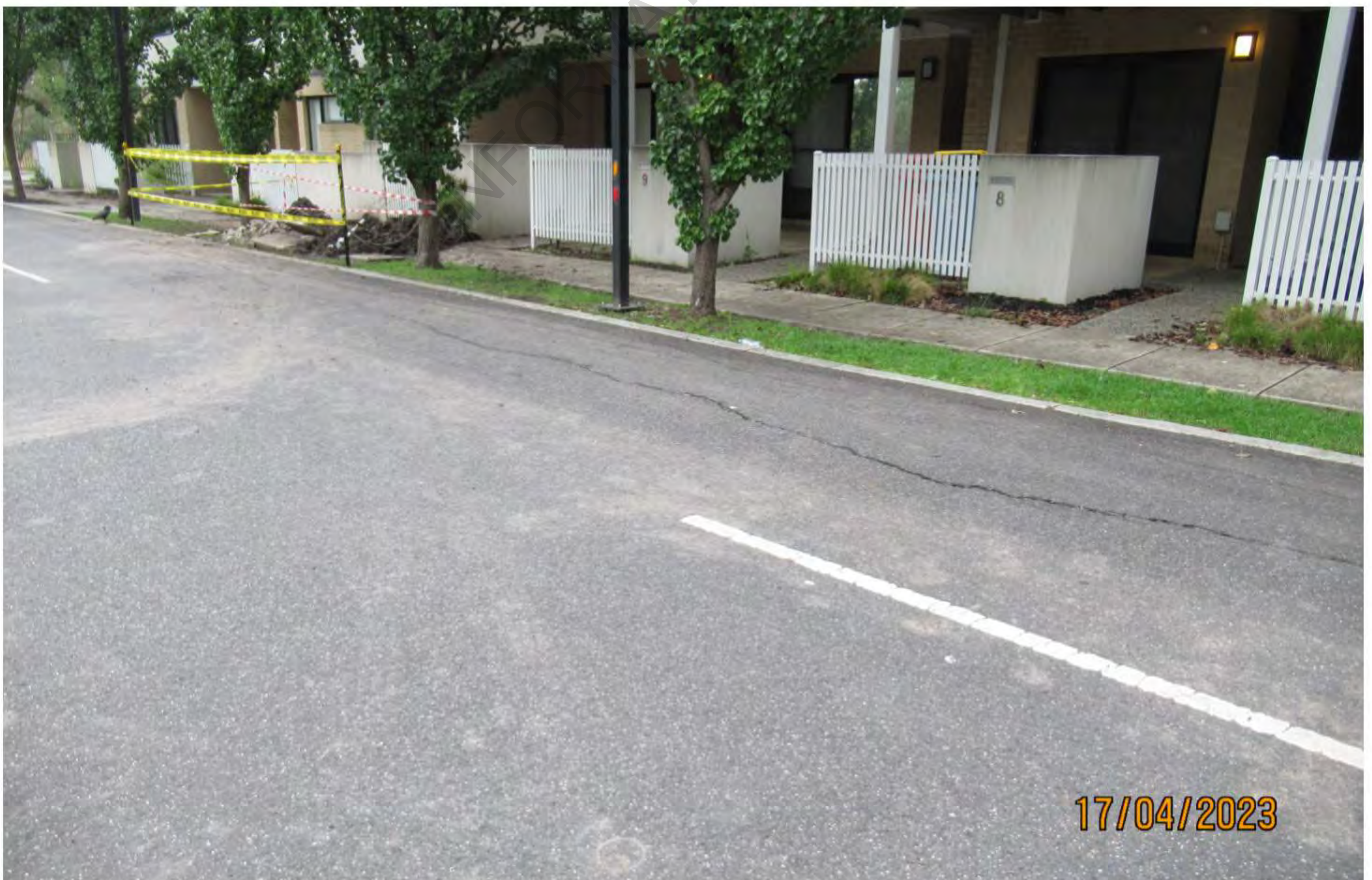
Photo 1.30: Increase in size and extent of longitudinal cracks in roadway
