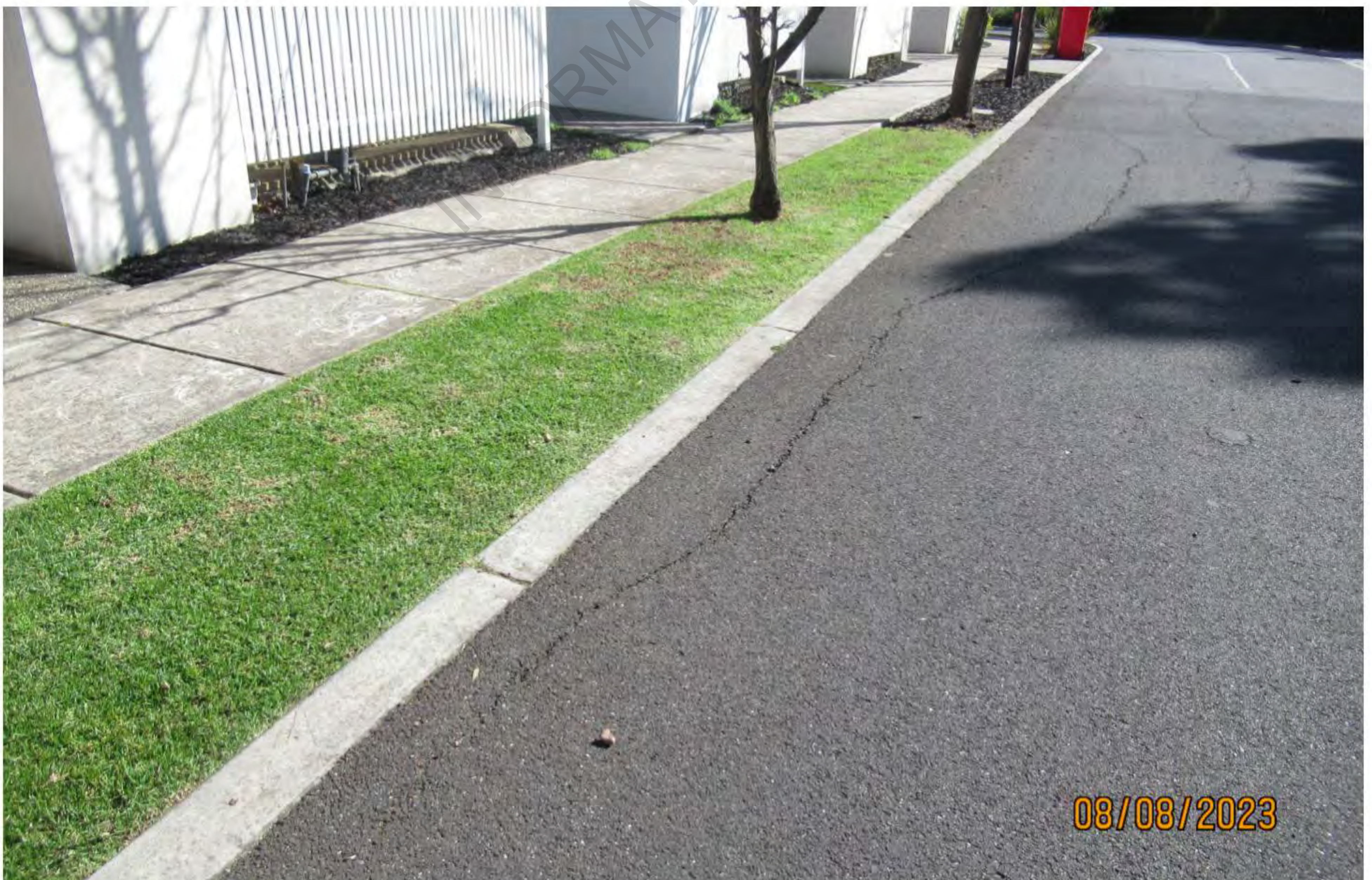
Photo 1.42: Cracking to roadway similar to that observed in April
