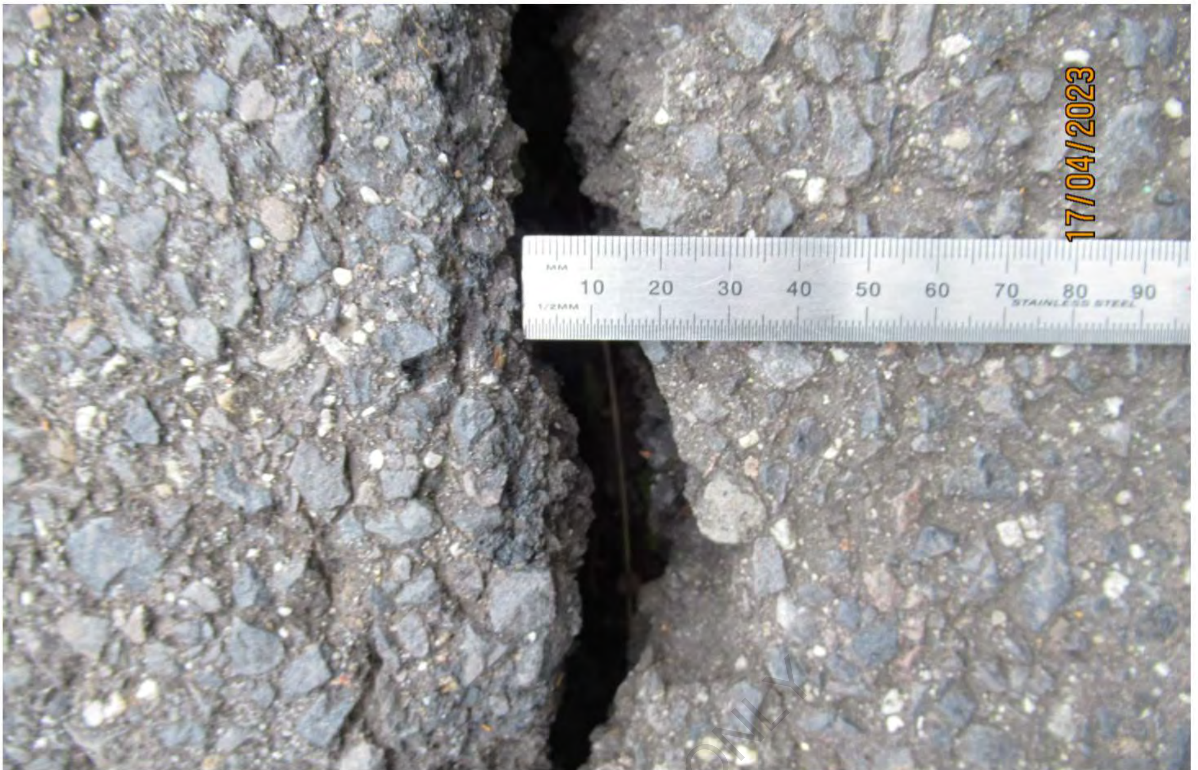
Photo 1.37: Measurement of crack width
