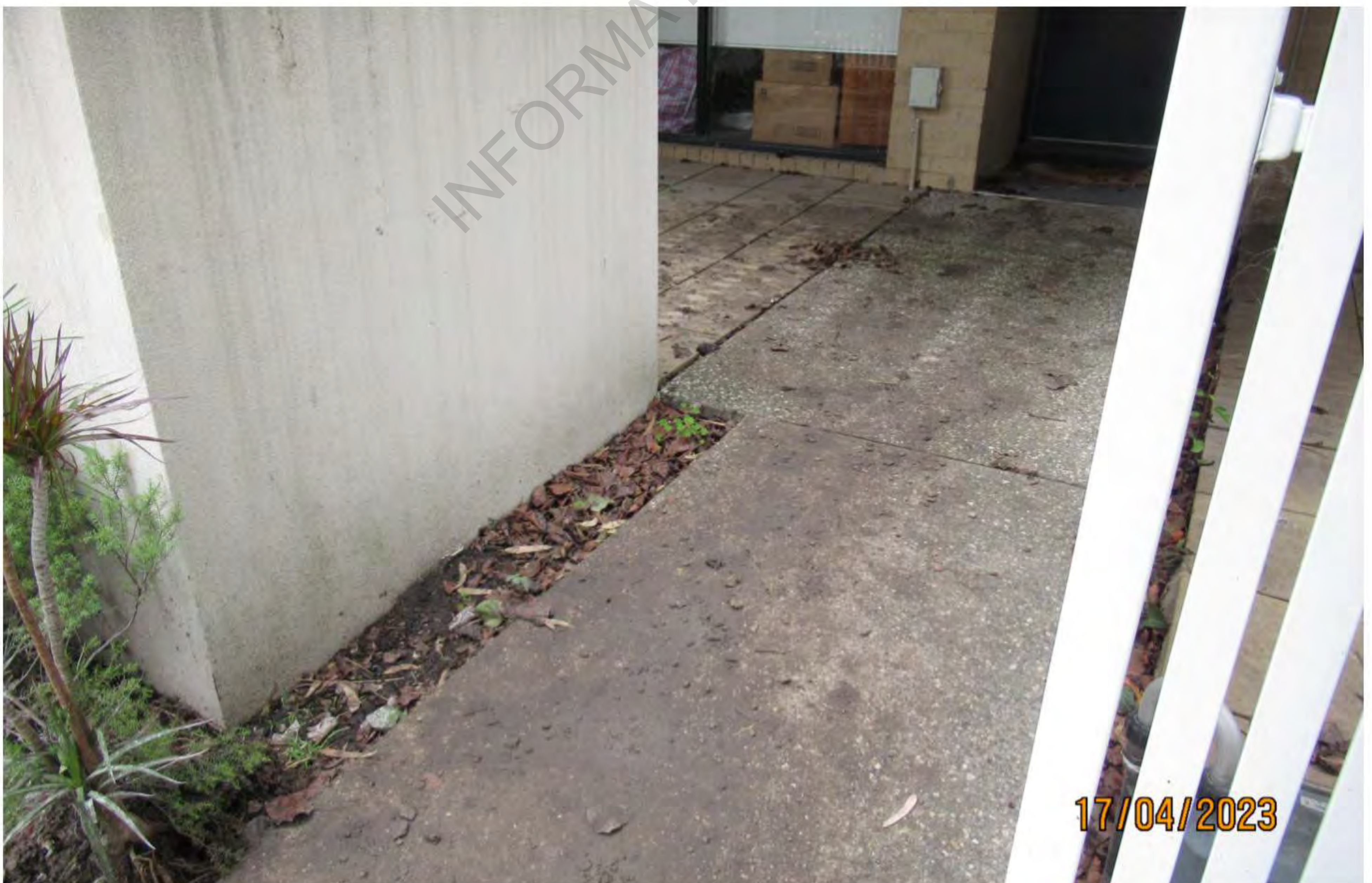
Photo 1.24: Visible signs of water inundation from leak
