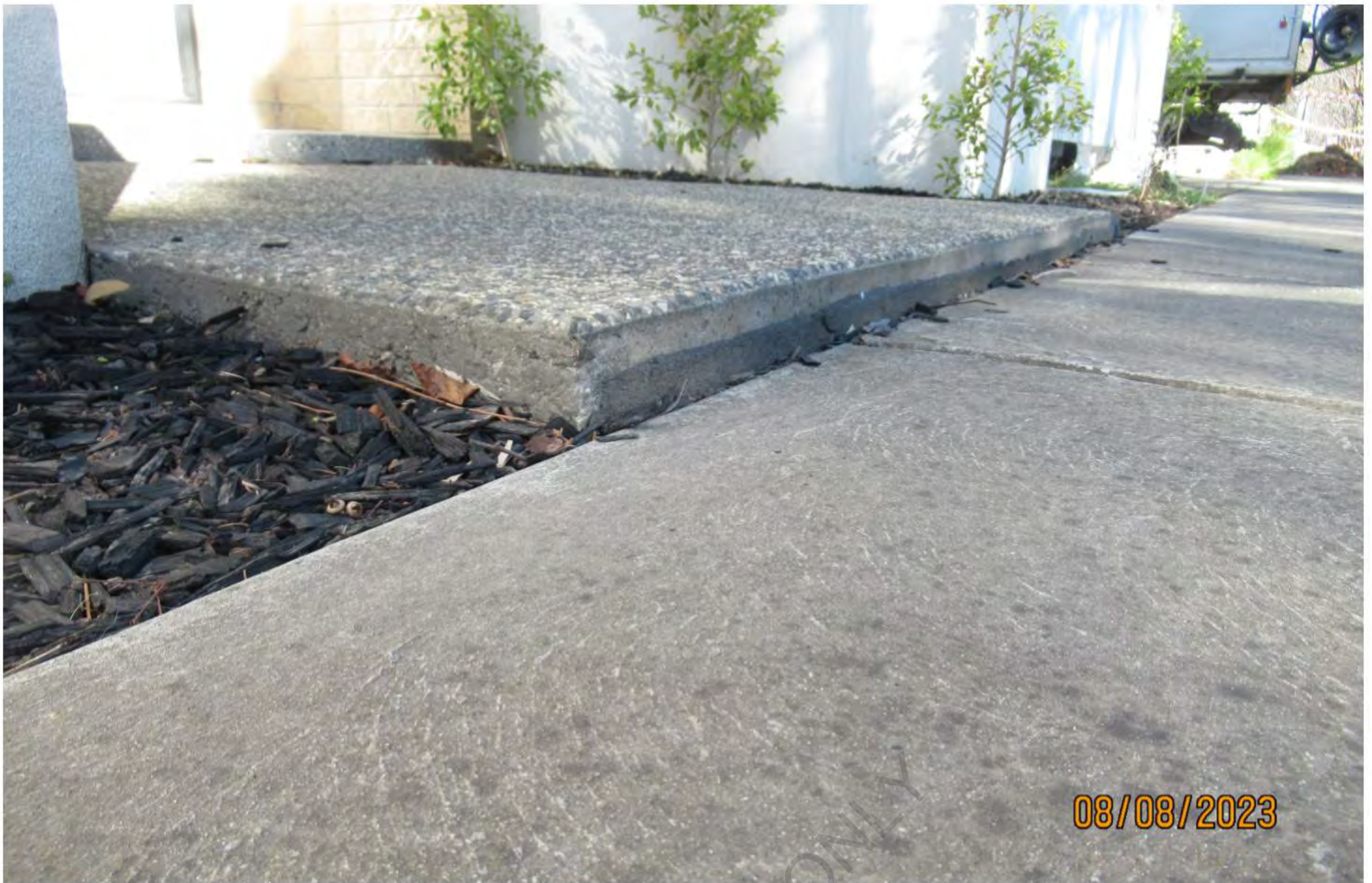
Photo 1.53: Differential settlement between footpath and townhouse pathway
