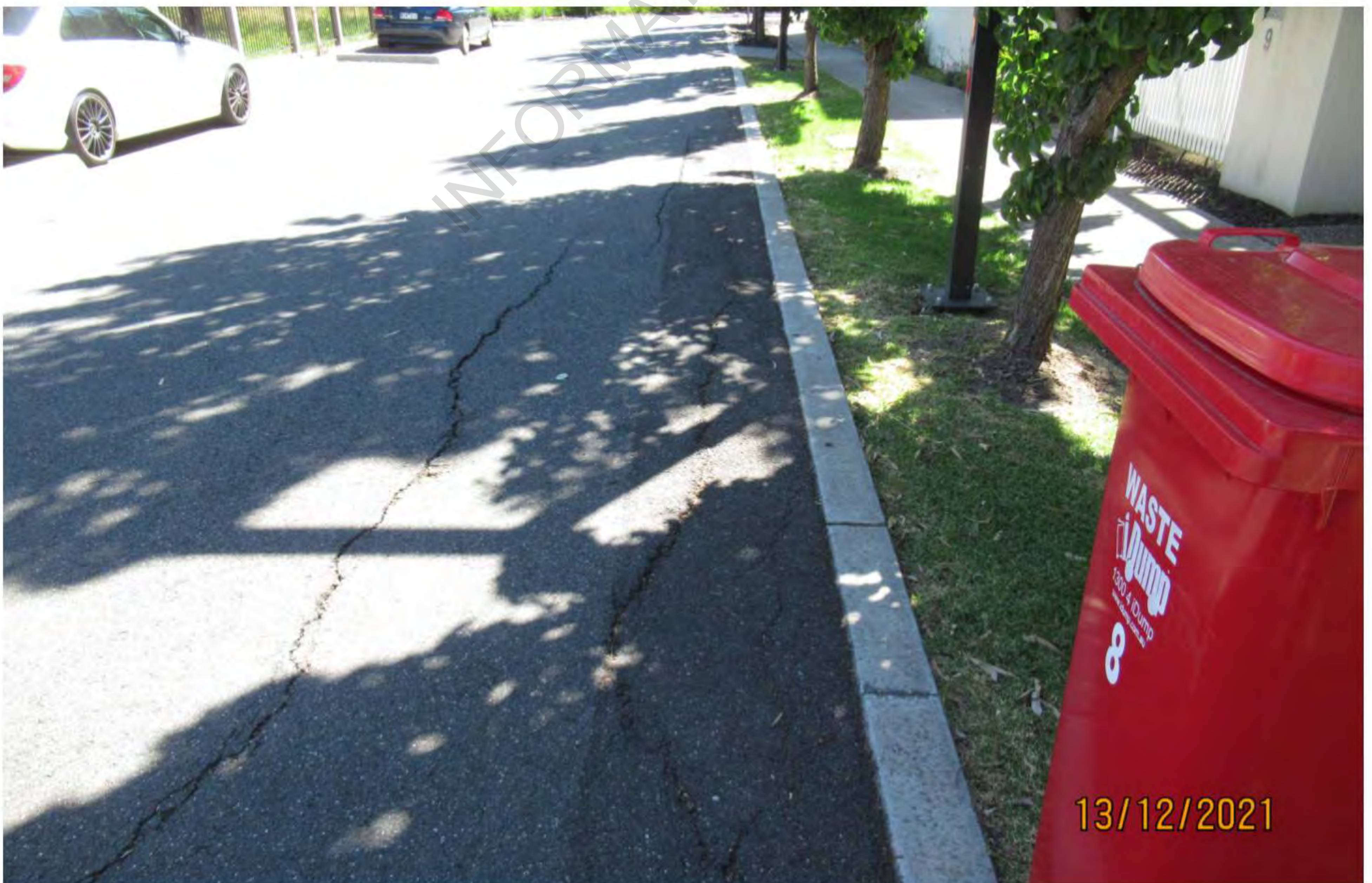
Photo 1.10: Longitudinal cracks in Leg A of Gorman Drive
