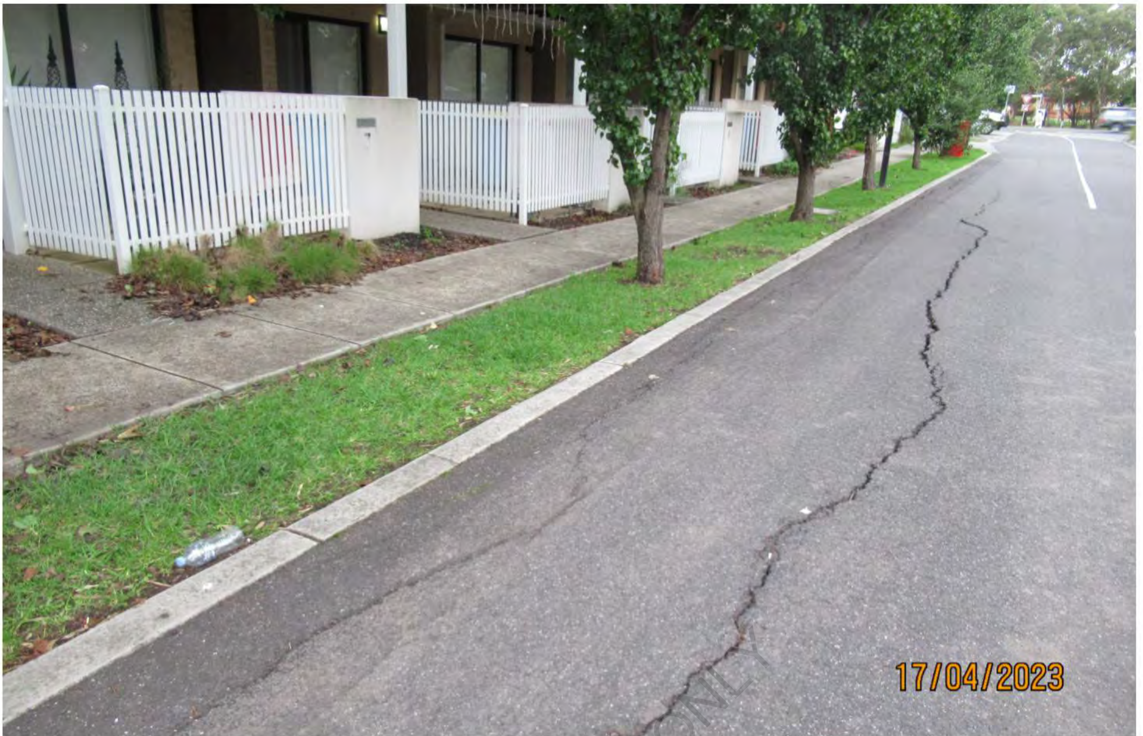
Photo 1.31: Increase in size and extent of longitudinal cracks in roadway
