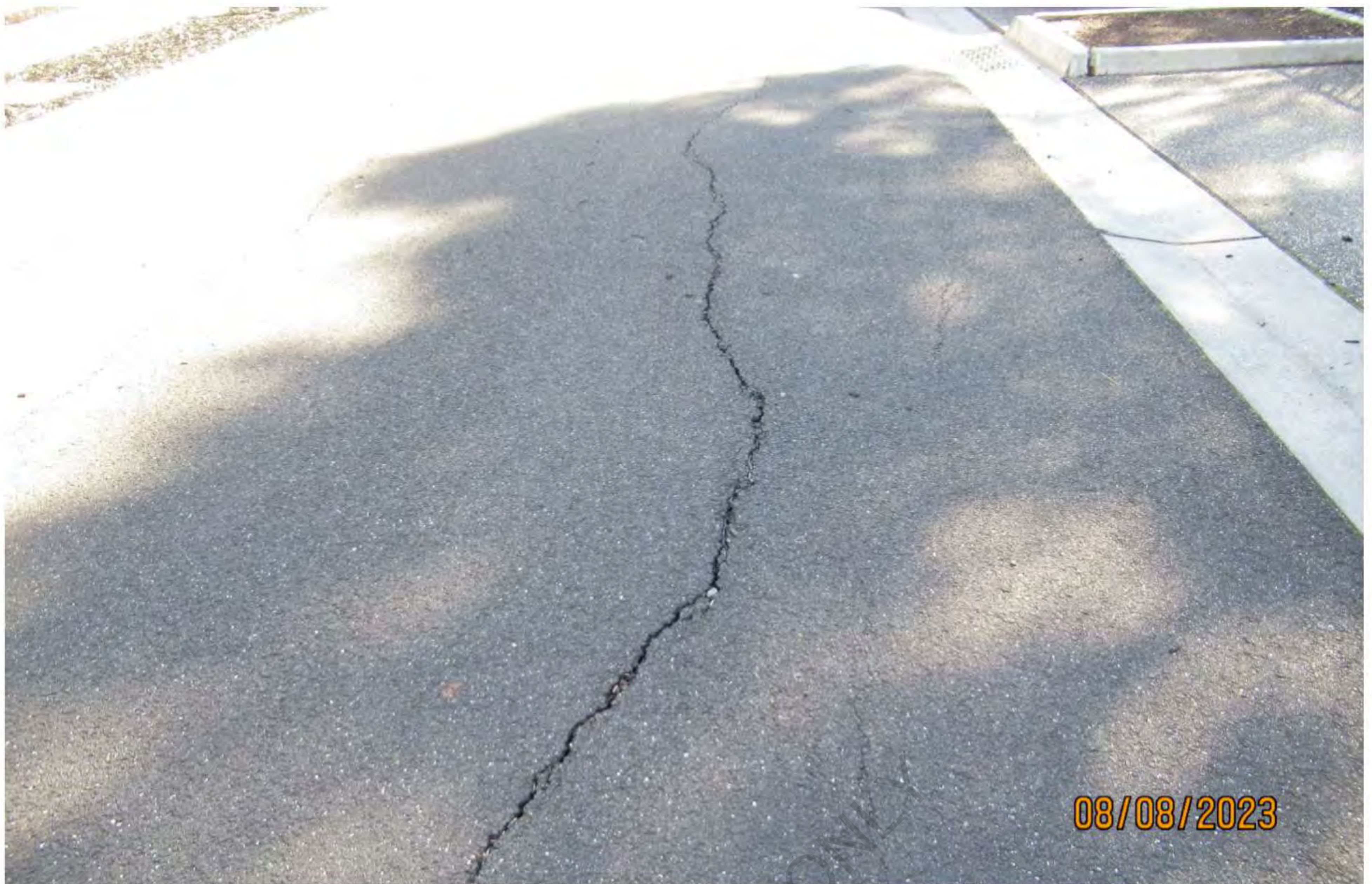
Photo 1.43: Cracking to roadway similar to that observed in April
