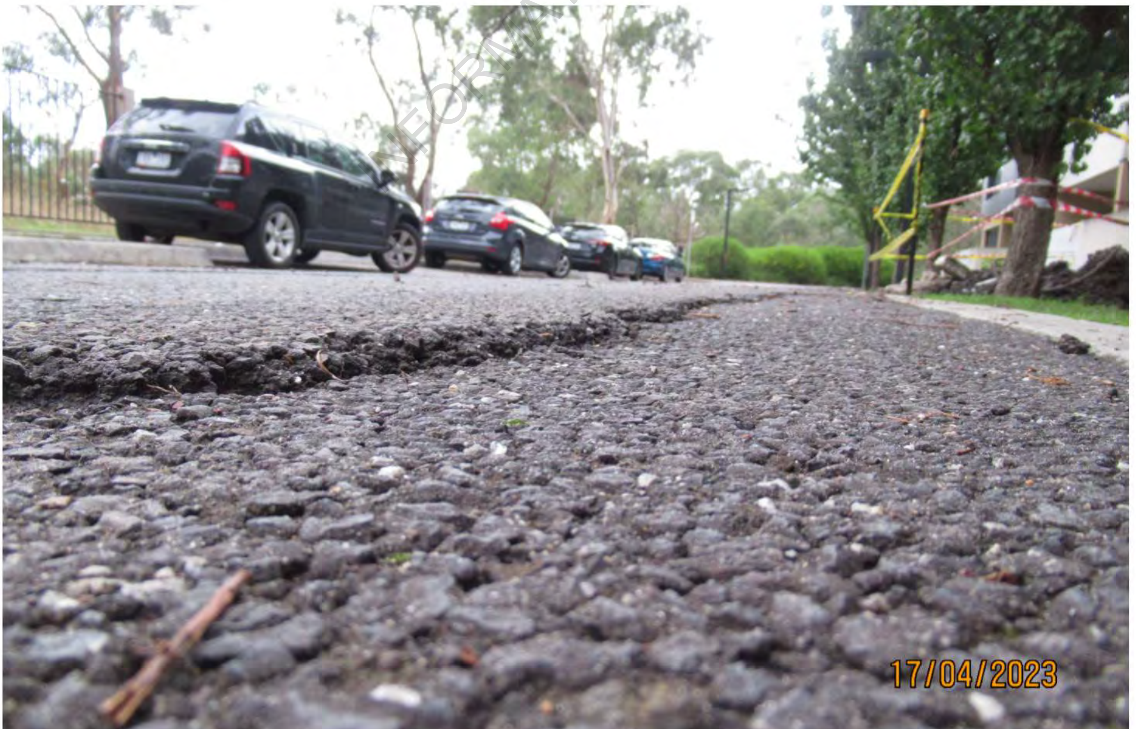
Photo 1.36: Displacement of the road surface across cracks had increased
