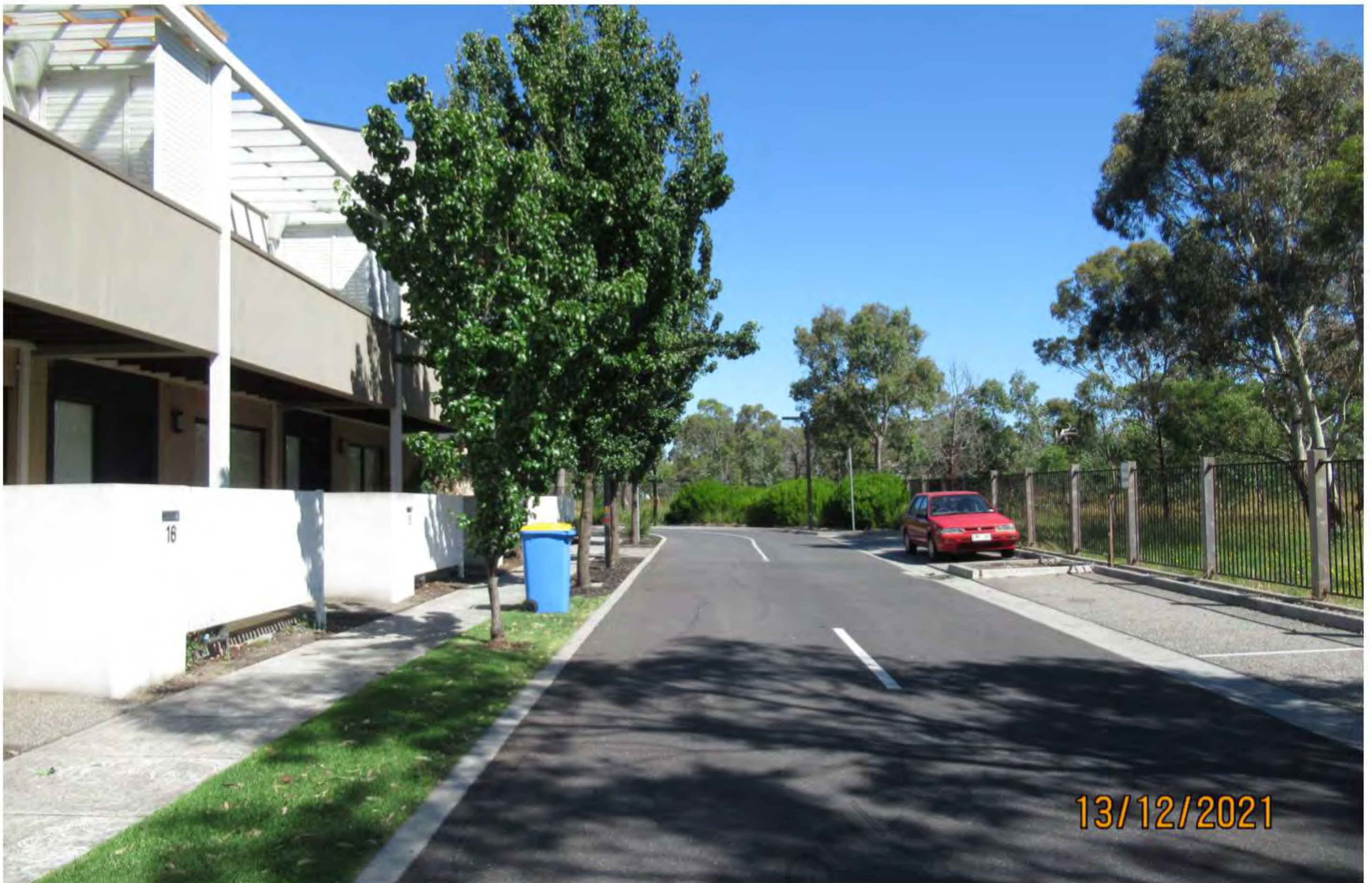
Photo 1.17: Longitudinal cracks in Leg B of Gorman Drive
