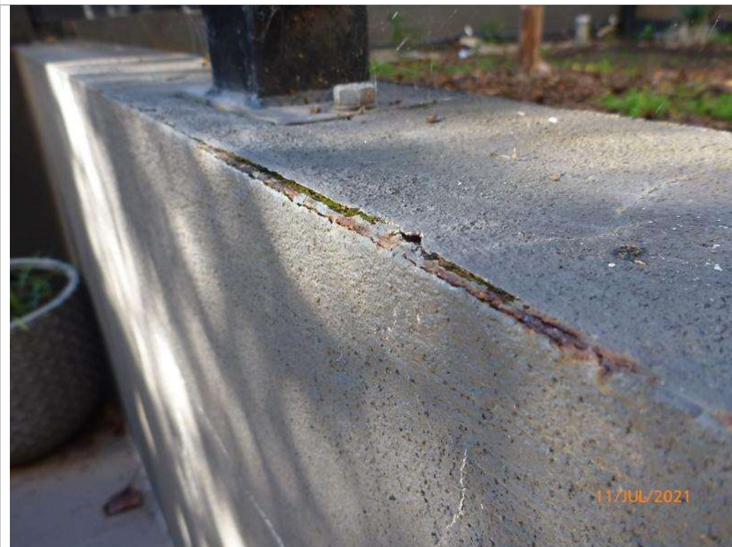
Photograph 30 – Rusted render corner beads
