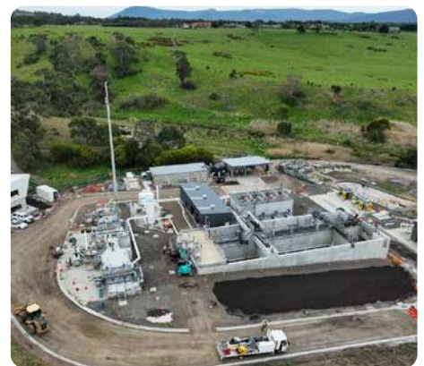
Gisborne Recycled Water Plant
