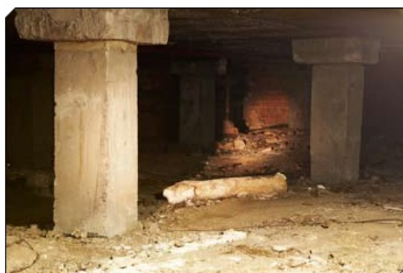
Figure 18: Unfixed asbestos lagging from a pipe.
