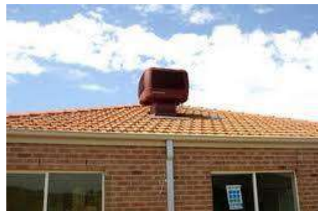
STANDARD UNIT IN CLEAR VIEW OF STREET NOT ACCEPTABLE
