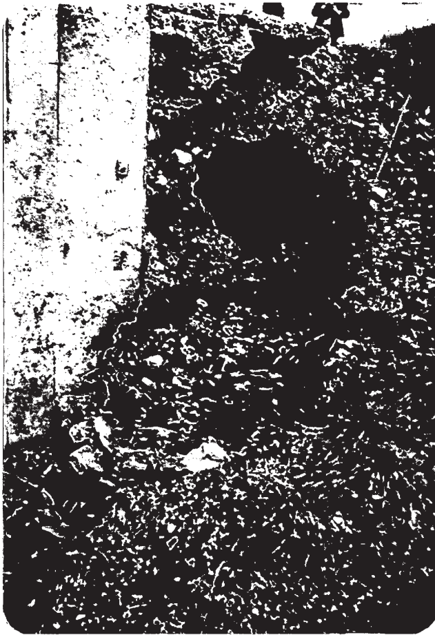
PLATE 20 - Undermining of a wingwall of the culvert shown in Plate 19.
