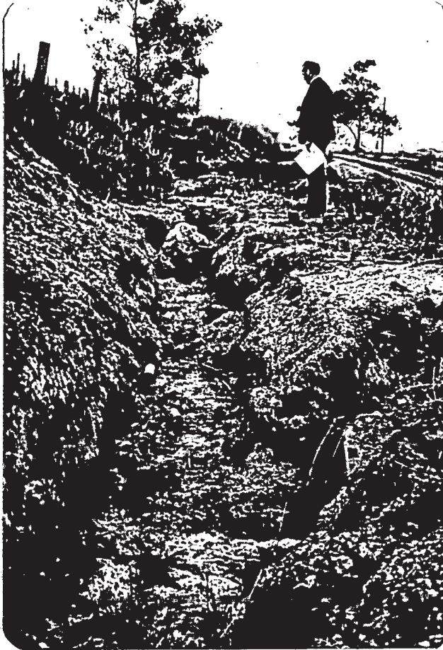
PLATE 4 - Roadside erosion along Seventh Avenue between Glenburnie Road and Second Avenue.
