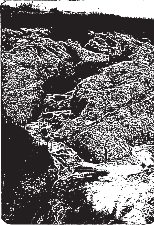
PLATE 16 - Bank degradation by overland flow (location on Plate 15). The shallow gully is probably the remnant of a collapsed tunnel. Fine sediment from the tunnels has been deposited on the gully floor.
