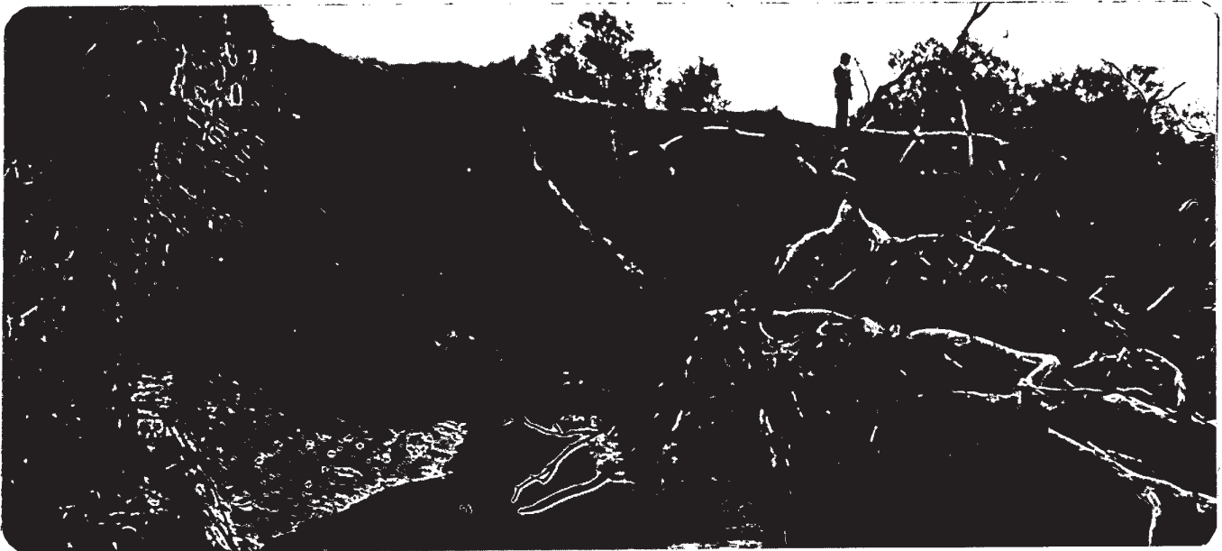
PLATE 2 - Undercutting on the outside of a bend along Barber's Creek.
