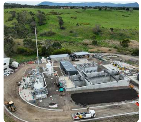
Gisborne Recycled Water Plant
