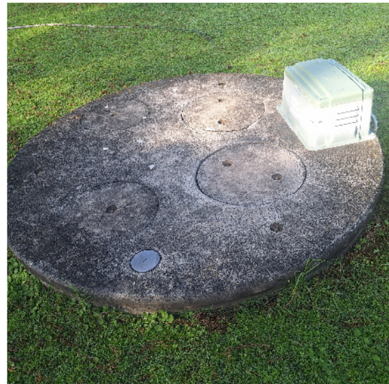
Photo 4: Existing secondary treatment system located on proposed Lot 2
